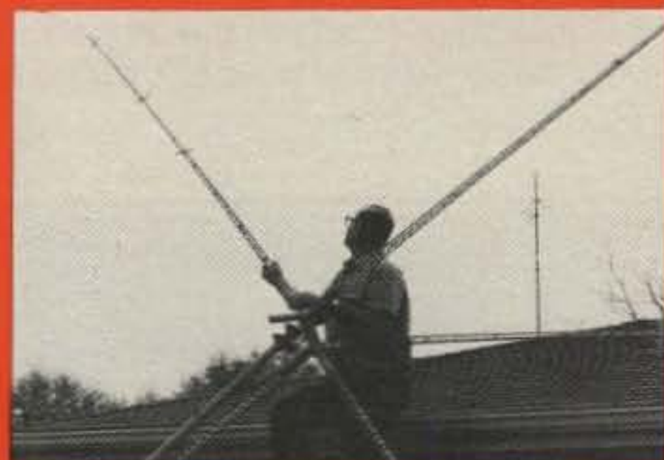
Hoisting the completed Gem-Quad into position on the house roof, ready to be shimmed up the mast using ropes and pulleys on the tower. Shown struggling with the array is Roy, WB4TKU.
