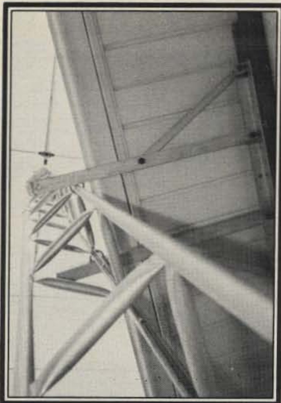
A close-up view of the tower mounting bracket which is bolted to the house.
