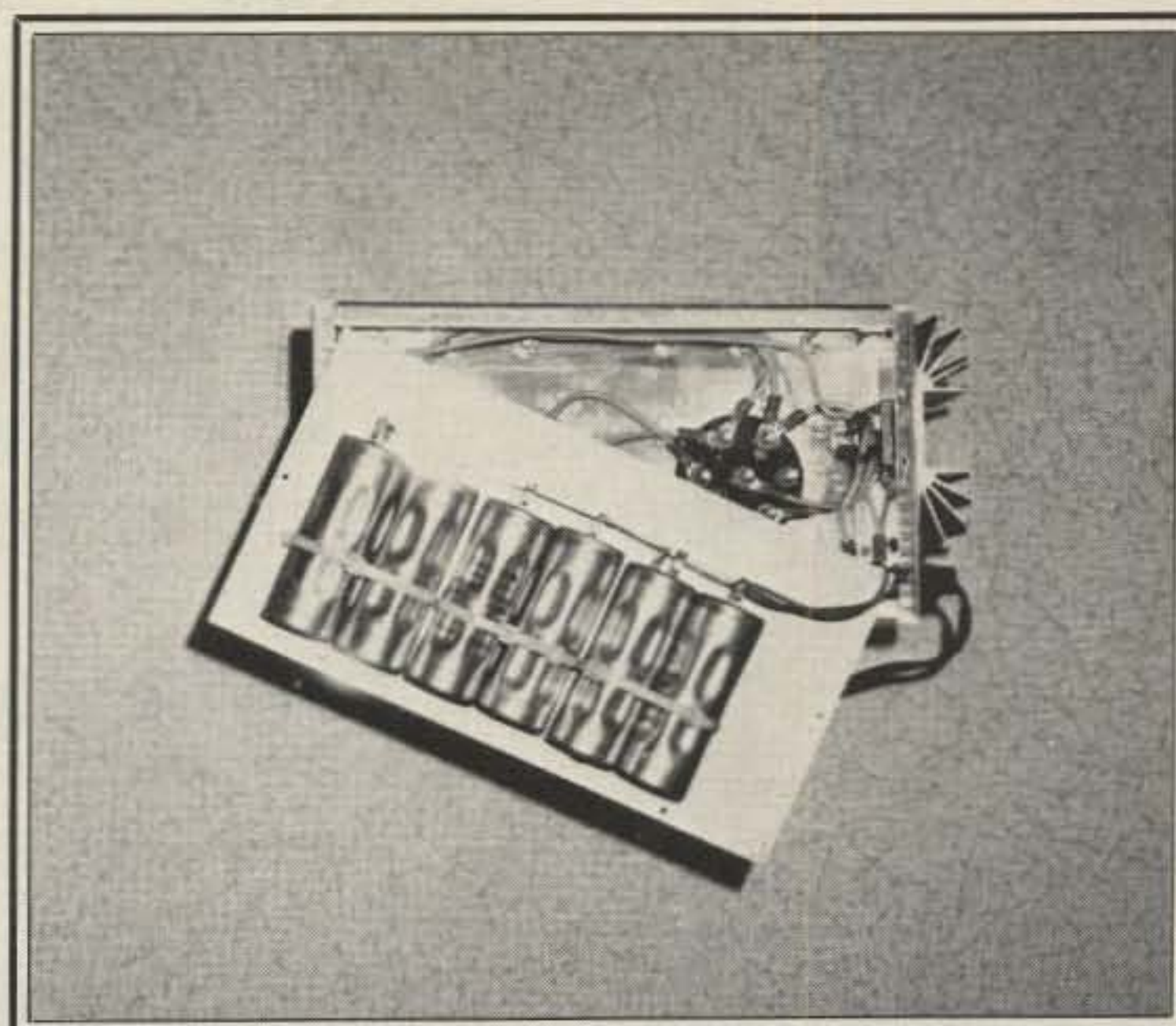
The six paralleled filter capacitors are held with tough plastic cable ties to the inside bottom plate of the power supply chassis.
