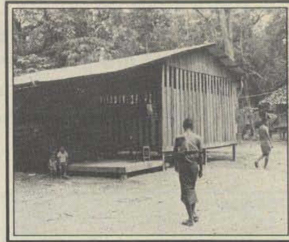
The man in the foreground with a rifle over his shoulder observes the raising of the beam in the back of the shack.
