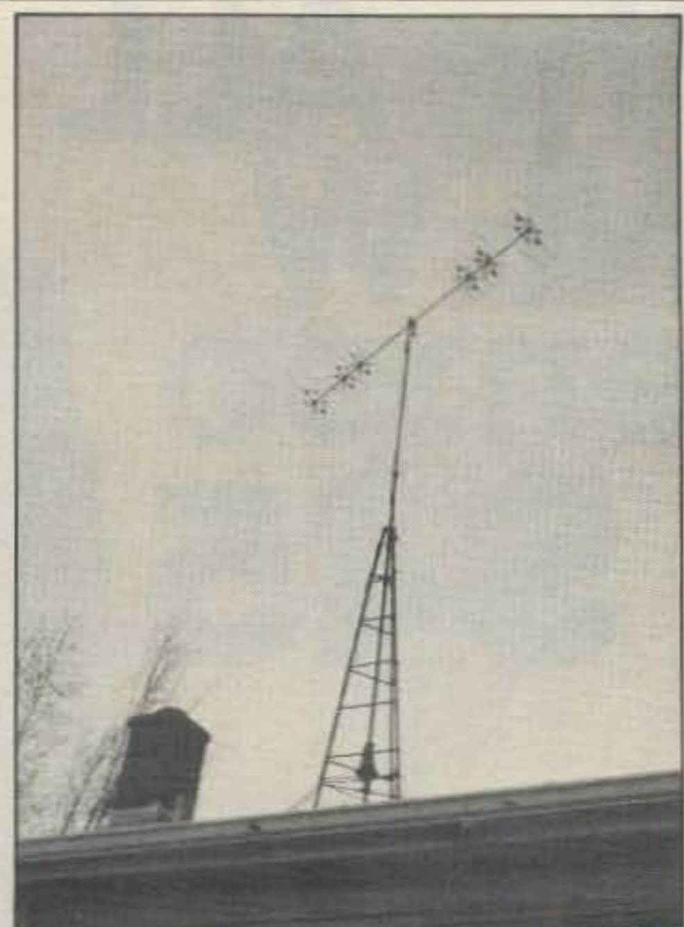
Fig. 6- The antenna is installed on a TV push-up mast mounted in a 10 foot tripod. The top of the tripod has been modified with a bearing and the entire mast rotates. The rotor is at roof-top level.
