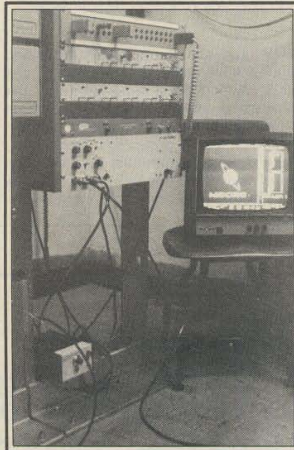
This is the head end of 1288 MHz ATV system used by W6ORG and W6VIO at JPL. Equipment includes circuit for superimposing call letters (W6ORG/W6VIO sequentially) on video from Voyager 2. Box on rack bottom is power supply and control unit for remote transmitter. Rest of rack gear is microwave and video distribution for JPL's TV system.
