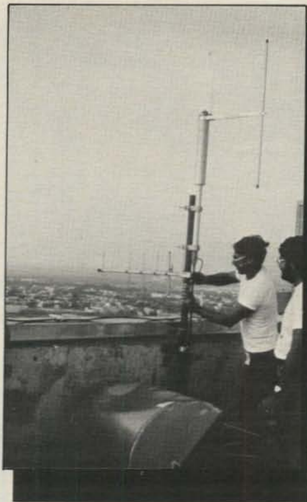
Fig. 2— SPARC installation team makes final adjustments to repeater antenna. (Left to right) Bot Stebbins, N2AAC, and Chuck Hewitt, WA2FQF. Taking photo was Nate Rosenthal, N2ADD. Also not shown, but a member of the team, was Charlie Rabey, N2CCR. Peeking between elements of the lower 450 MHz link antenna is Atlantic City's "far out" casino, Harrah's. Far out, that is, in their being the only casino in town not to be located at the Boardwalk. In fact, they aren't even on the Monopoly board.
