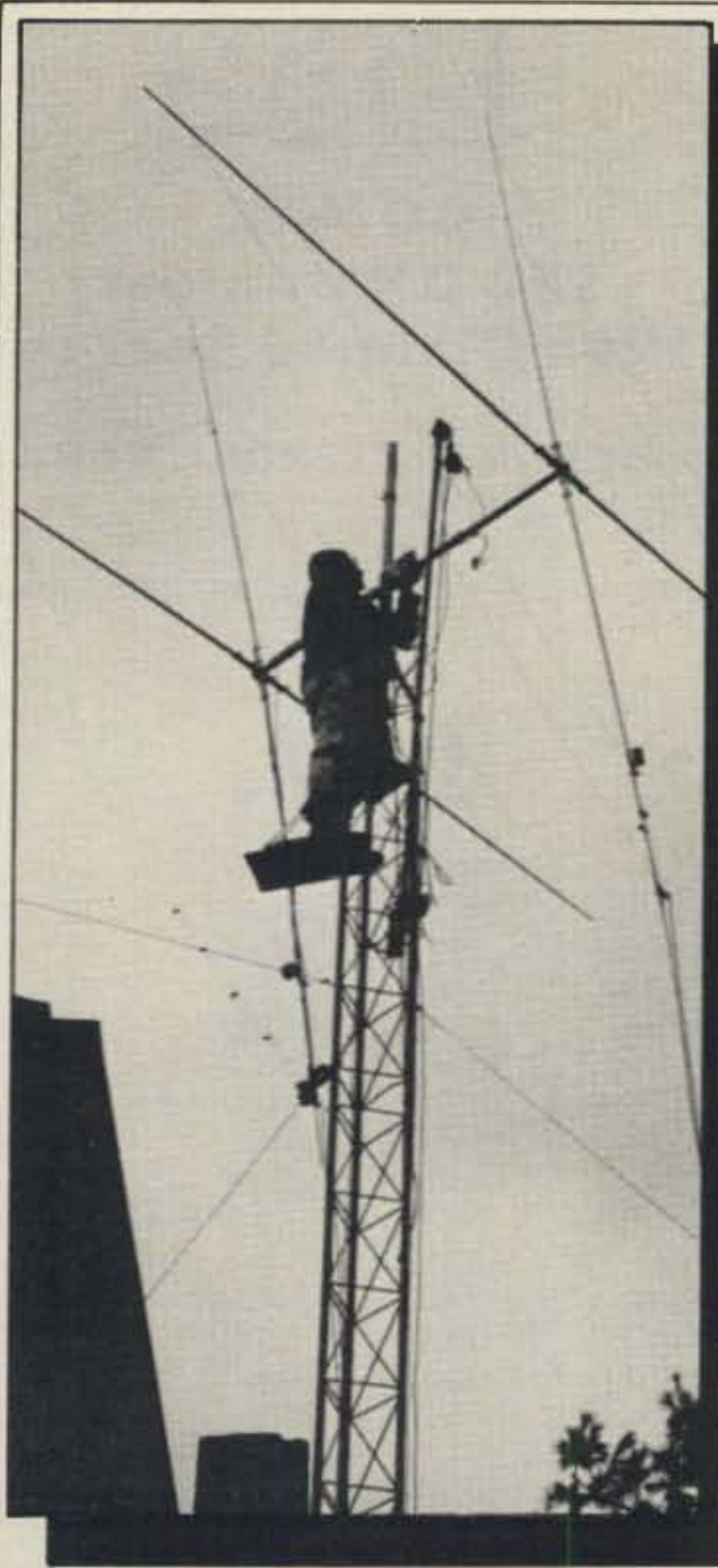
Antenna has been swung 90° out from under the boom and is being secured to the rotating mast temporarily to drop the boom before final tightening.
