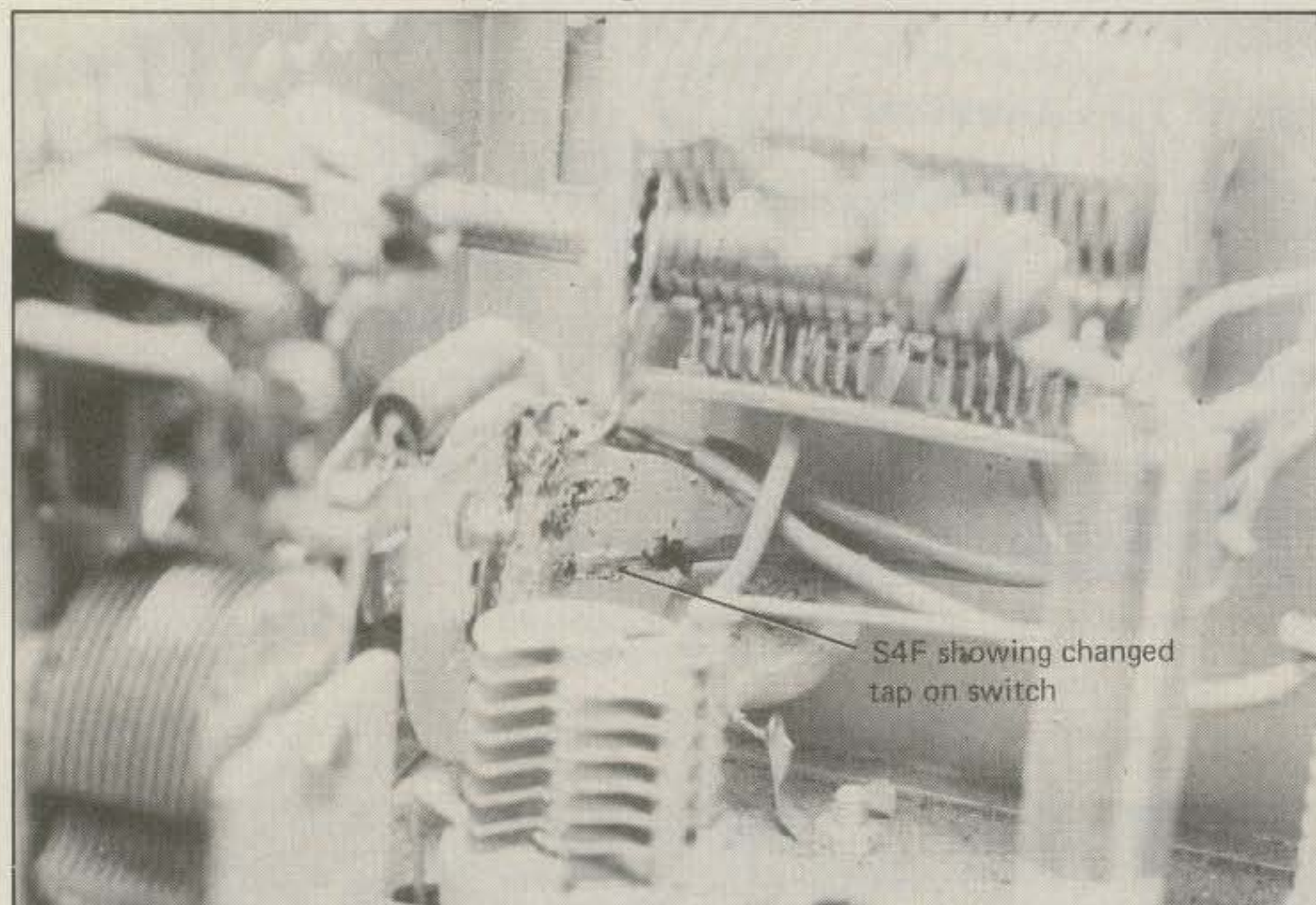
A close-up view of S4(F) showing the changed tap on the bandswitch.
