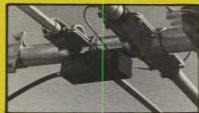
Feed point and balun
