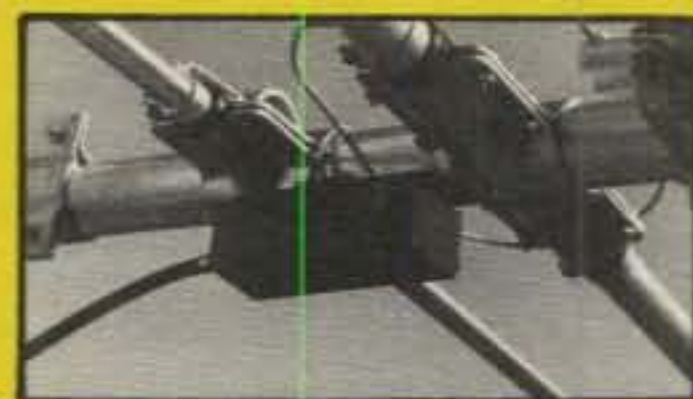
Feed point and balun
