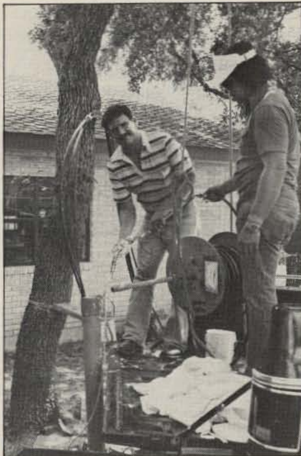
Duane Price, WB5VWX, and Craig Kennedy, KB5BI, of Kennedy Associates, Inc., feed Andrews Hardline into the underground duct with the aid of a lot of cable soap.
