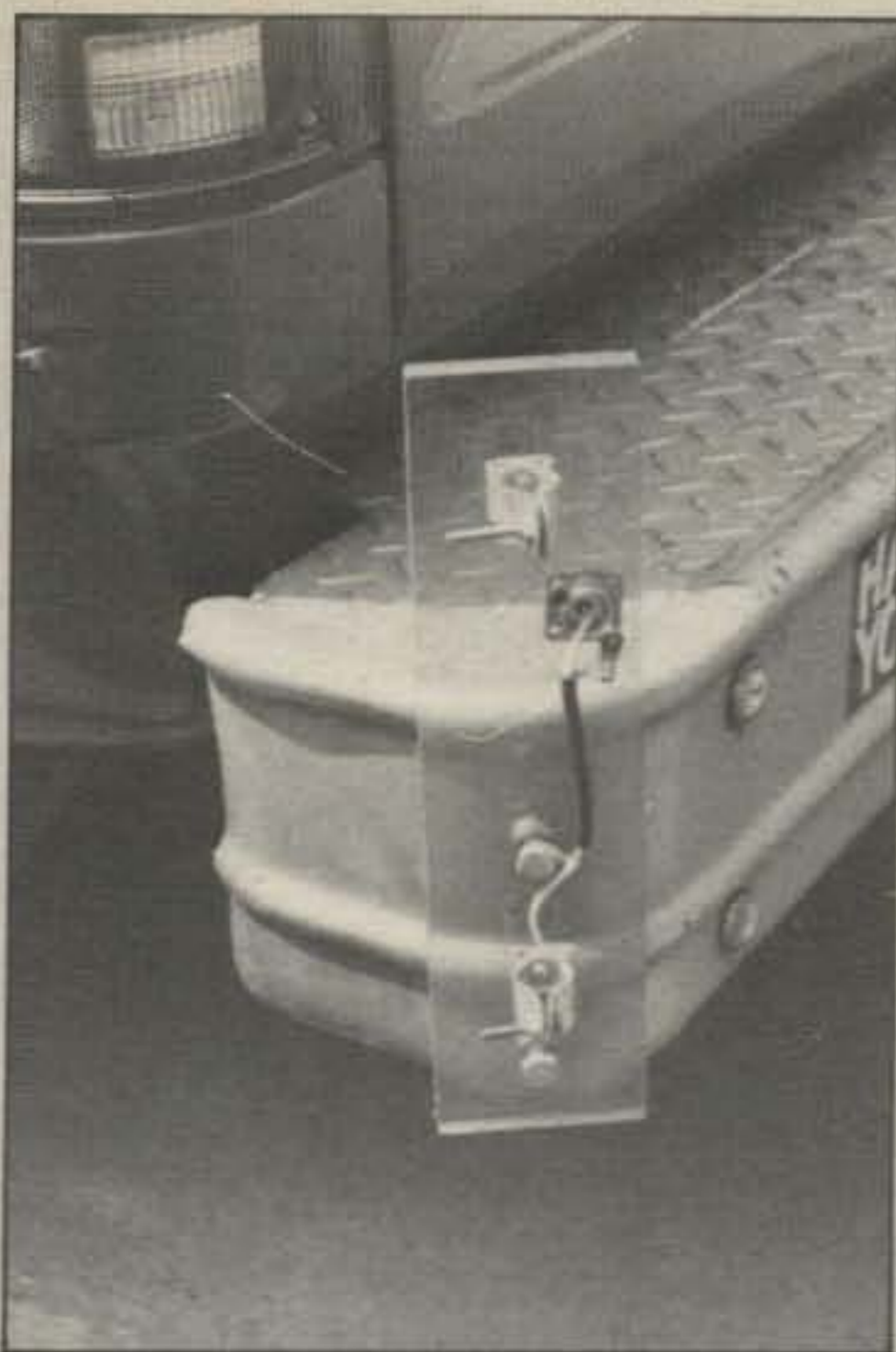
The conduit is held in place by conduit clips as shown.
