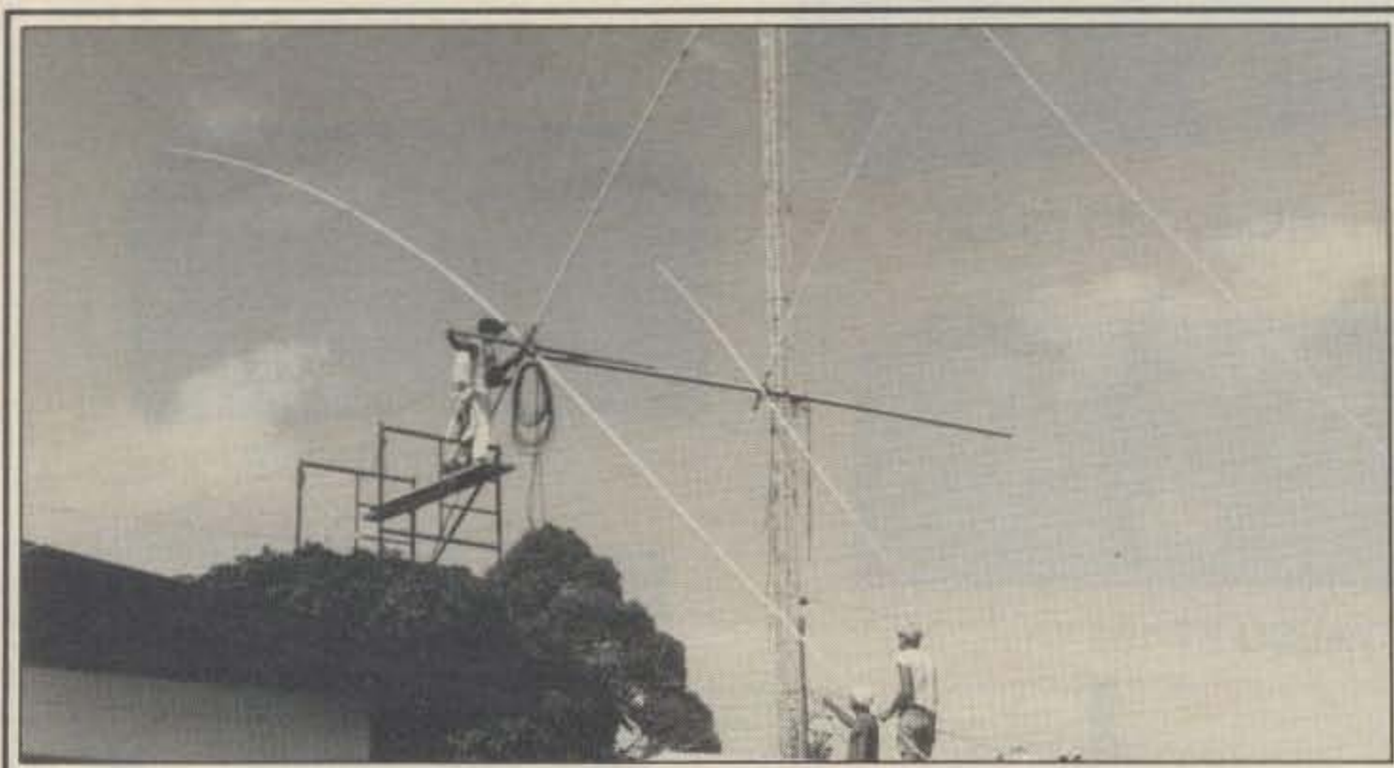
This shows the installation of the first monster element (10 meter third director, 15 and 20 meter directors, 40 meter driven element). At the opposite end of the boom is a support cable.
