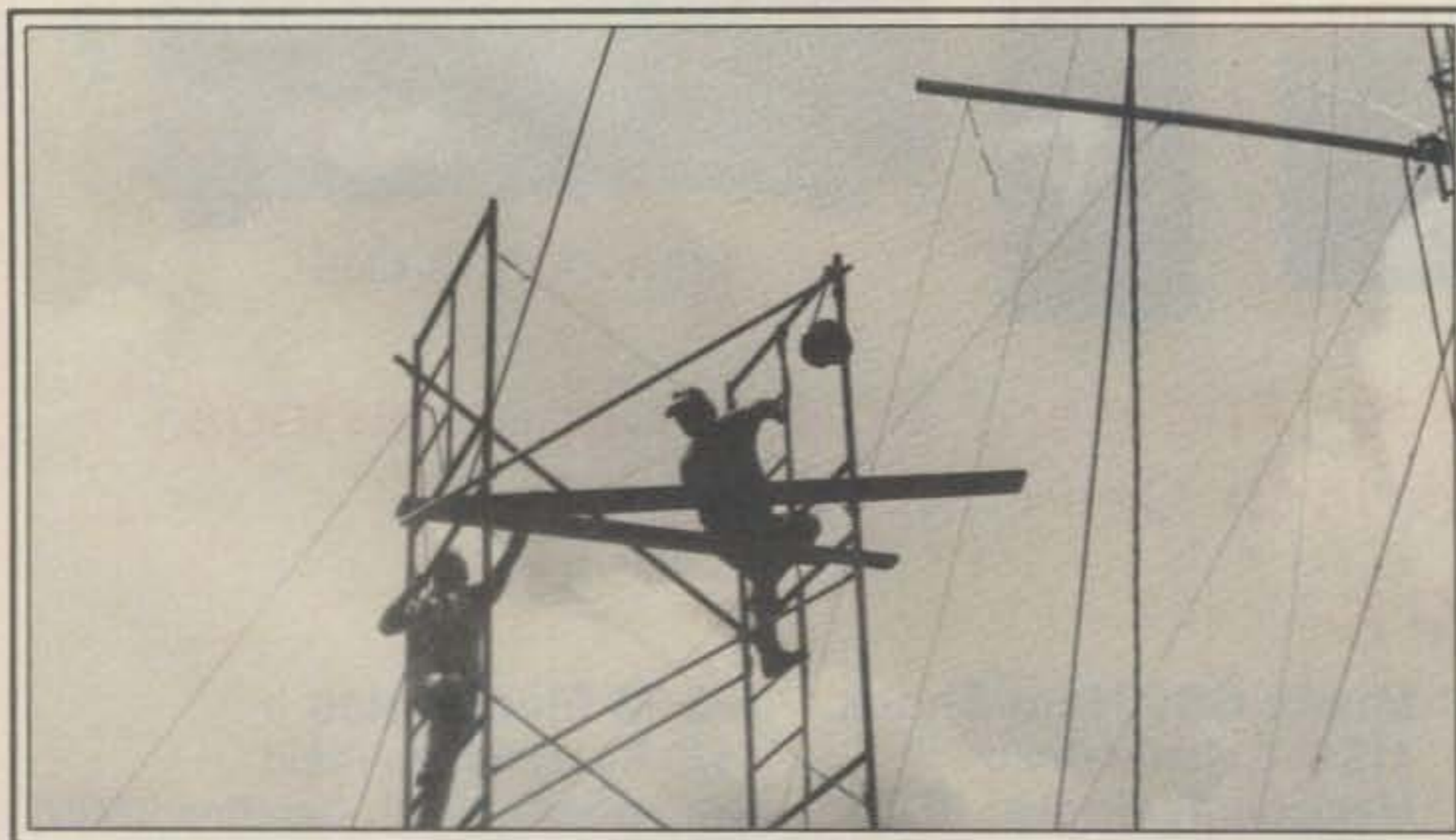
The scaffolding had to be moved to the other end of the boom. Note that for safety's sake the scaffolding is guyed.
