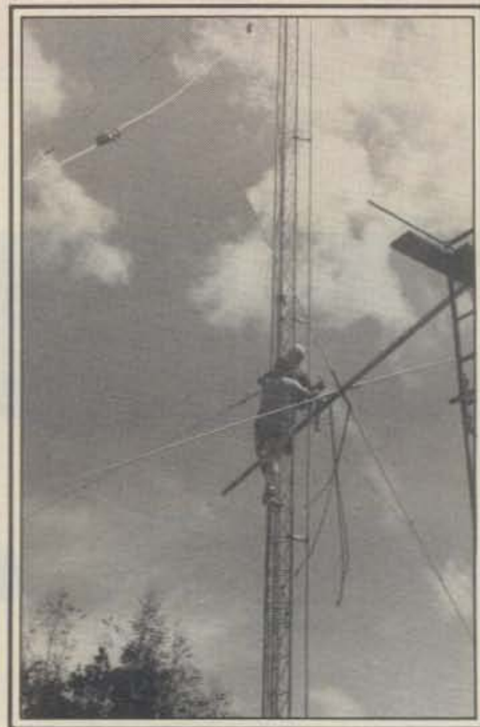
Here is a closeup of that installation. Note the elevator rail on the tower.
