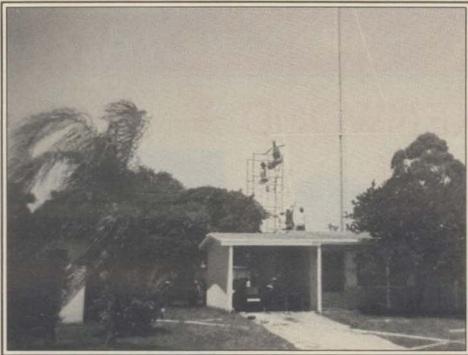
The scaffolding is erected, and installation commences with the middle element (10 meter first director, 15 and 20 meter driven elements).
