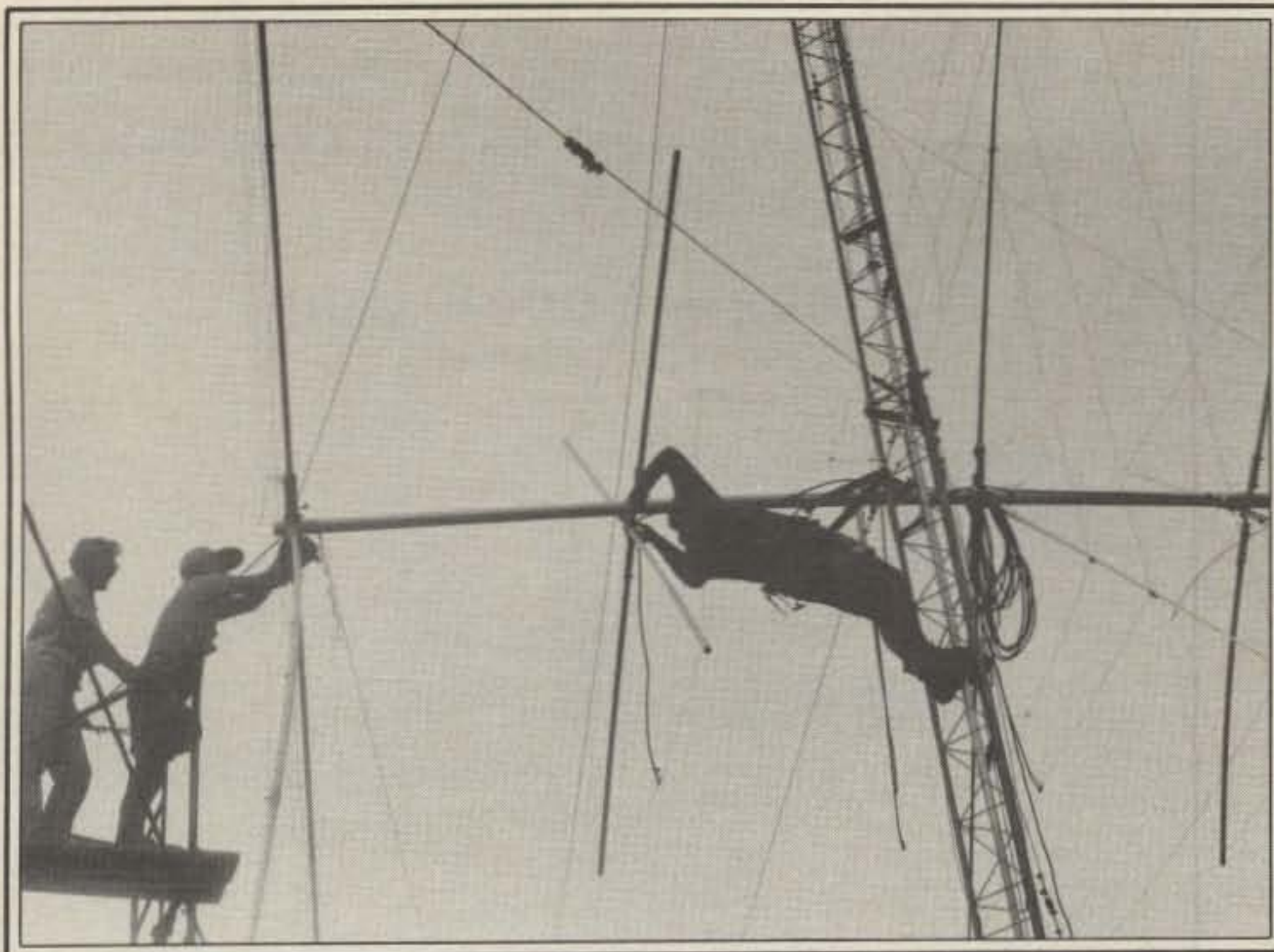
Here are the final two elements being installed. The only way to attempt the acrobatics I performed is with a heavy-duty lineman's belt.
