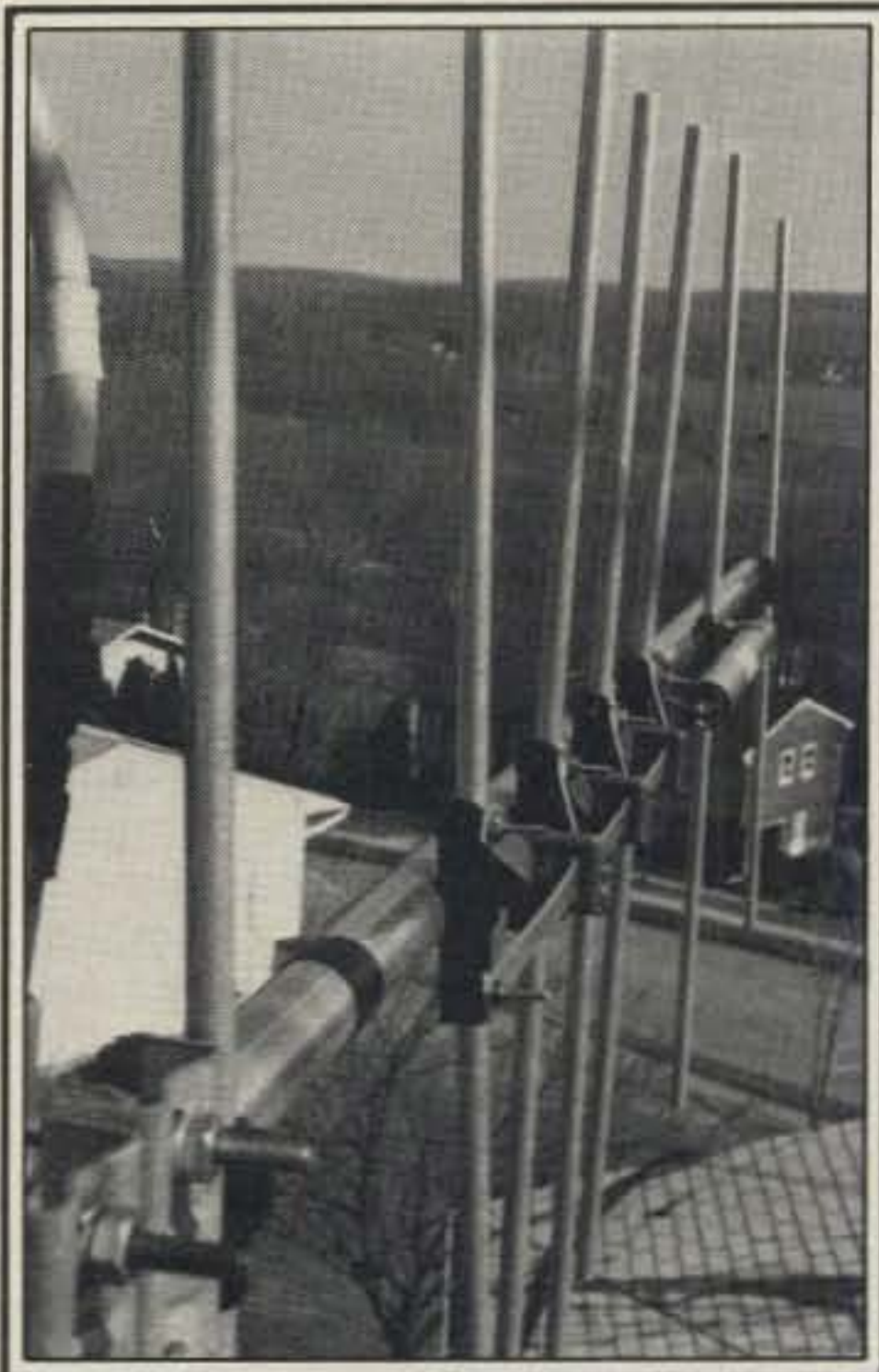
The right way to install a vertically-polarized beam antenna: end-mounted to a tower leg behind its reflector element. Shown is a KLM 7-element Yagi with log-periodic feed system and "sleeve" balun. This is the 220 MHz "link" antenna at WB2WIK/R.
