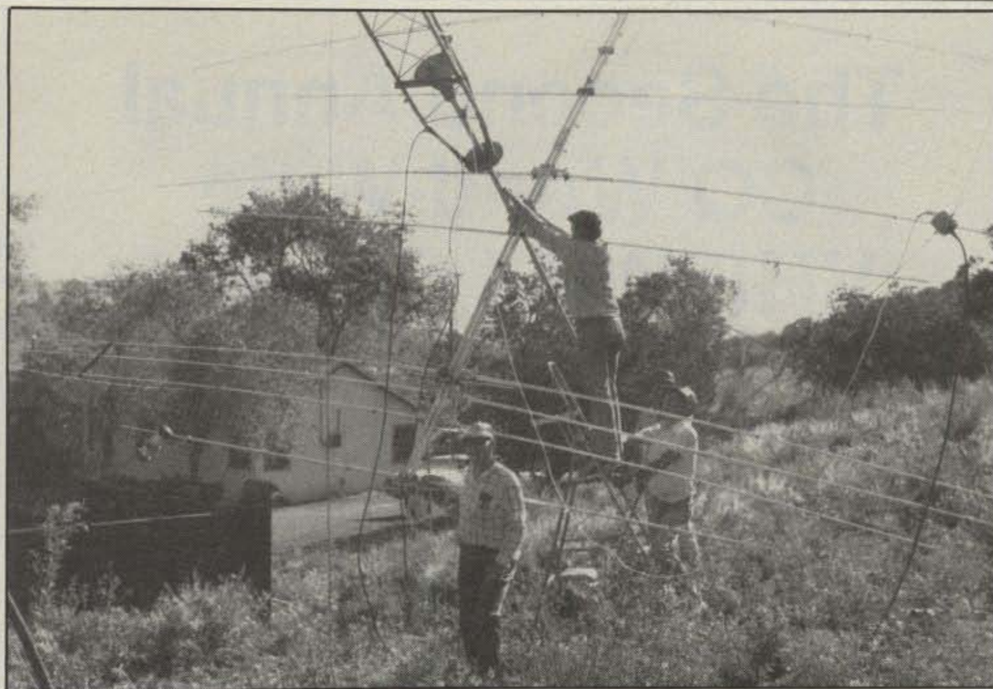
I have a Rohn Model 45 crank-over, and it proved to be no easy job getting the beam on mast—in the upside-down position. However, with the help of some intrepid local amateurs, we got the job done.
