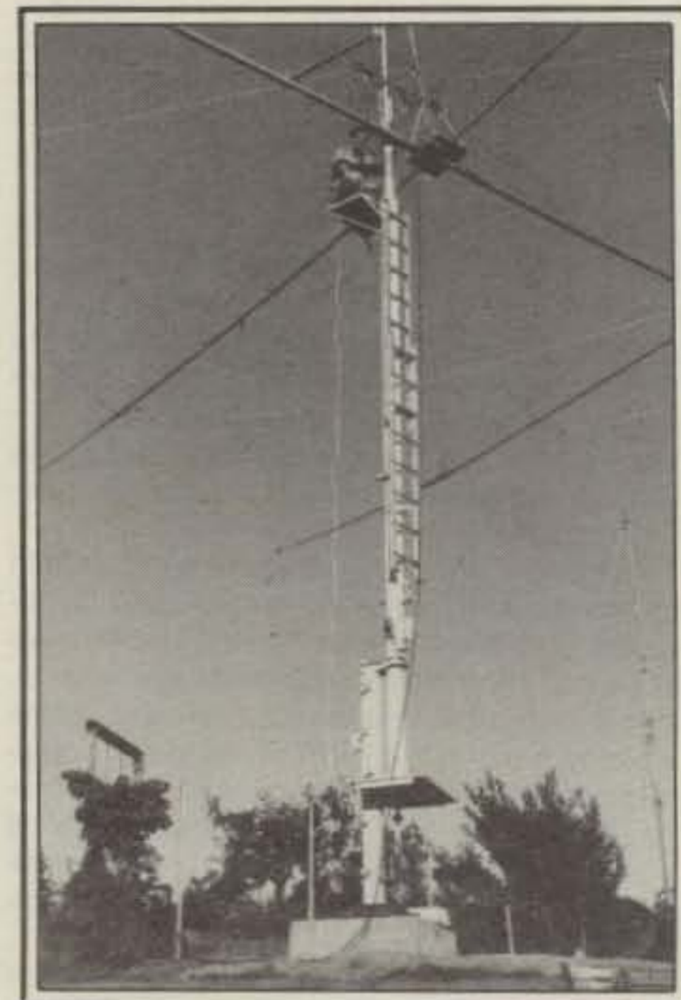
N7AM Quad installation showing the first base used. The base had to be reengineered after complications arising from damage in a severe windstorm. The new base is considerably stronger and more rigid.
