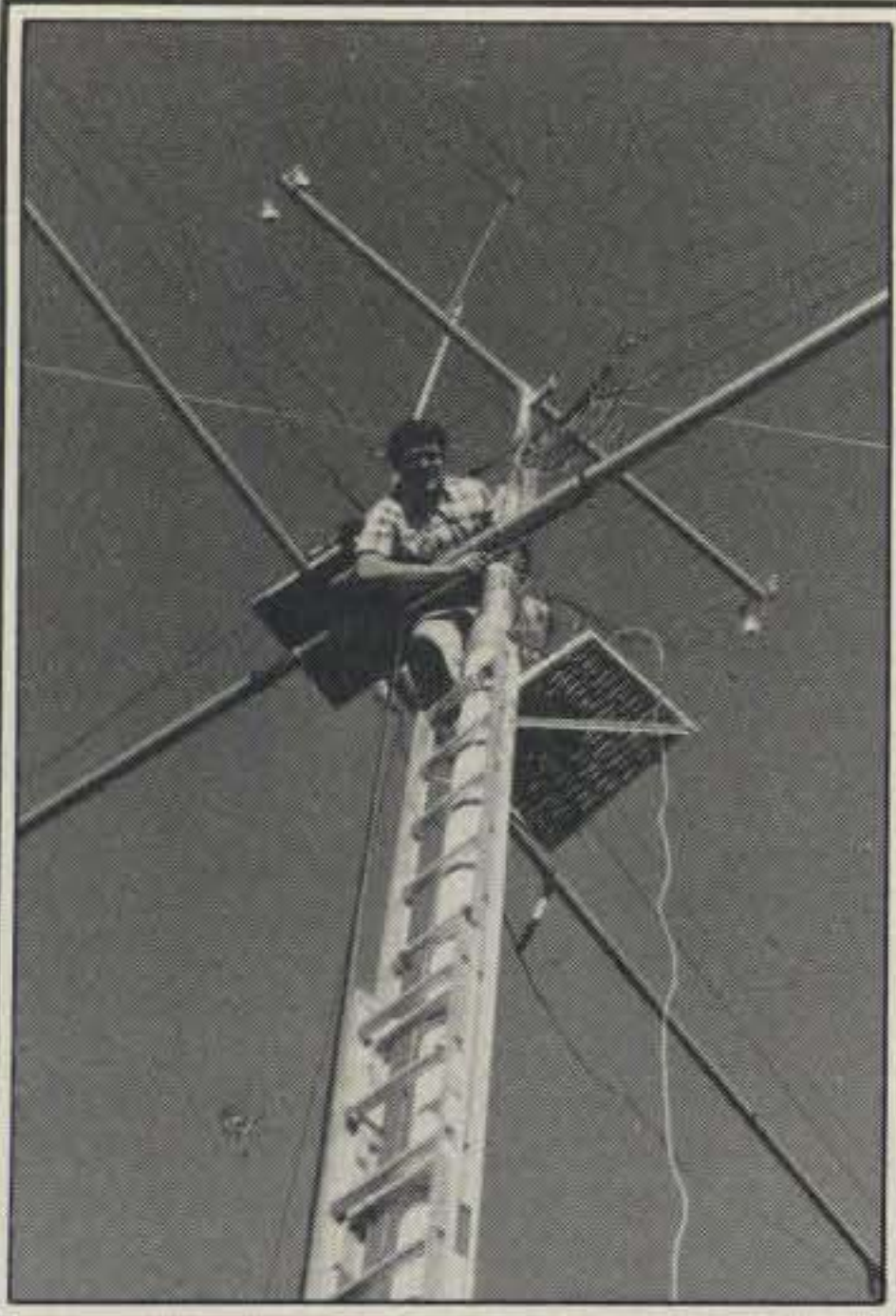
N7AM Quad installation showing Jerry, NC7U, getting the topside work done in order to be able to get the lateral guys attached to the boom.
