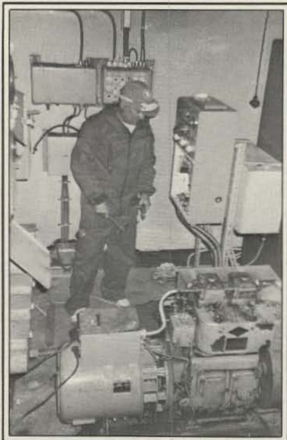
The Market Reef Electricity Company Unlimited was responsible for a solid supply of 6 kw of power, using a diesel generator ferried by a chopper. OHØRJ did a superb job.
