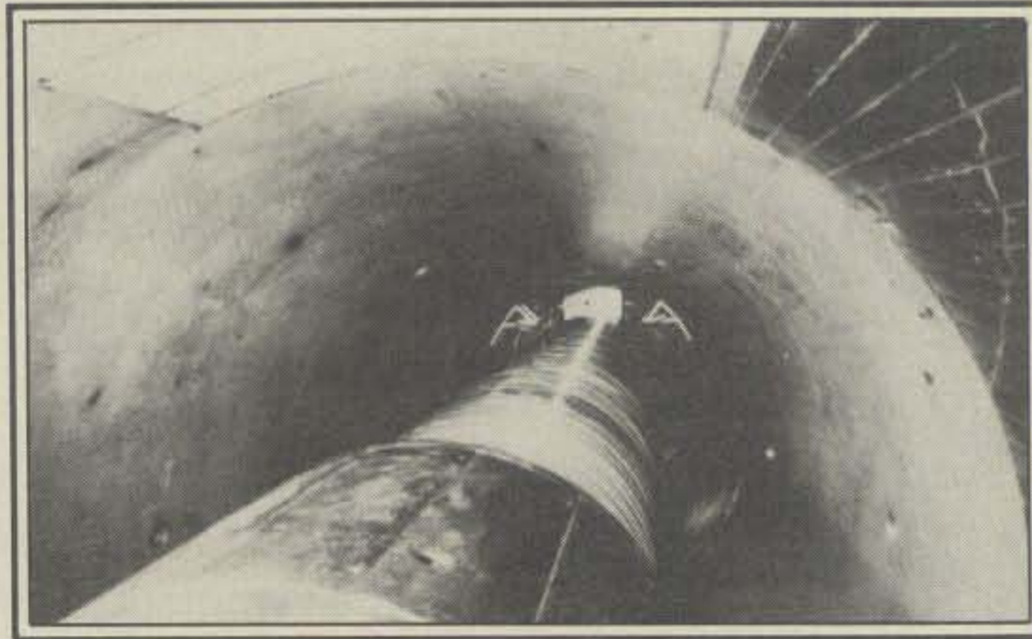
Inside the high-voltage tank. It's an eerie place. The high-voltage terminal in the foreground is about as large as a small automobile. The column rings, which obscure the pelletron chains and the beam tube, ensure a uniform voltage gradient throughout the acceleration process. (Photo courtesy Univ. of Rochester Nuclear Structure Research Lab)
