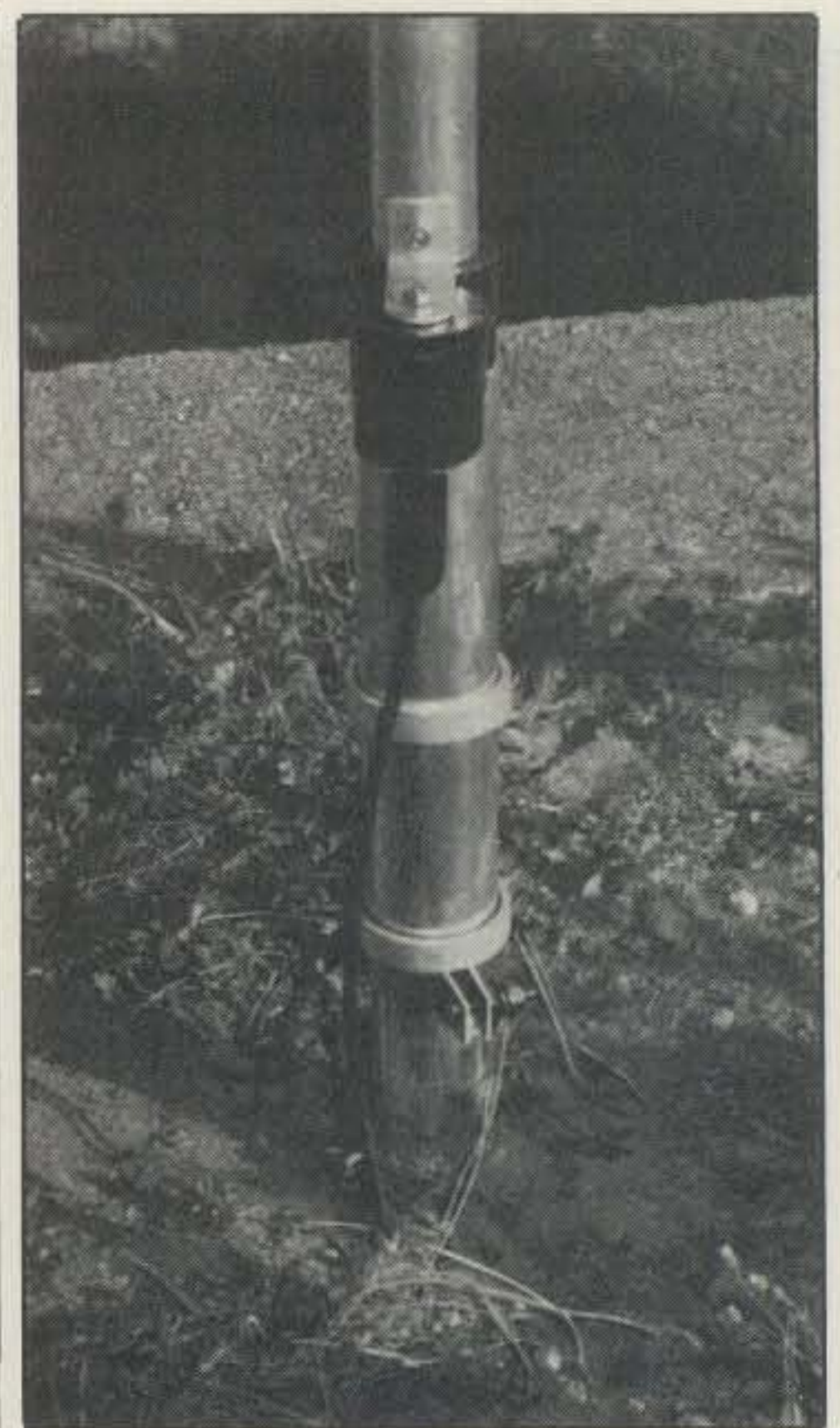
In this installation, the base of the AP8 has been placed over one end of a four foot section of 1 3/4" aluminum tubing which has been driven into the ground.
