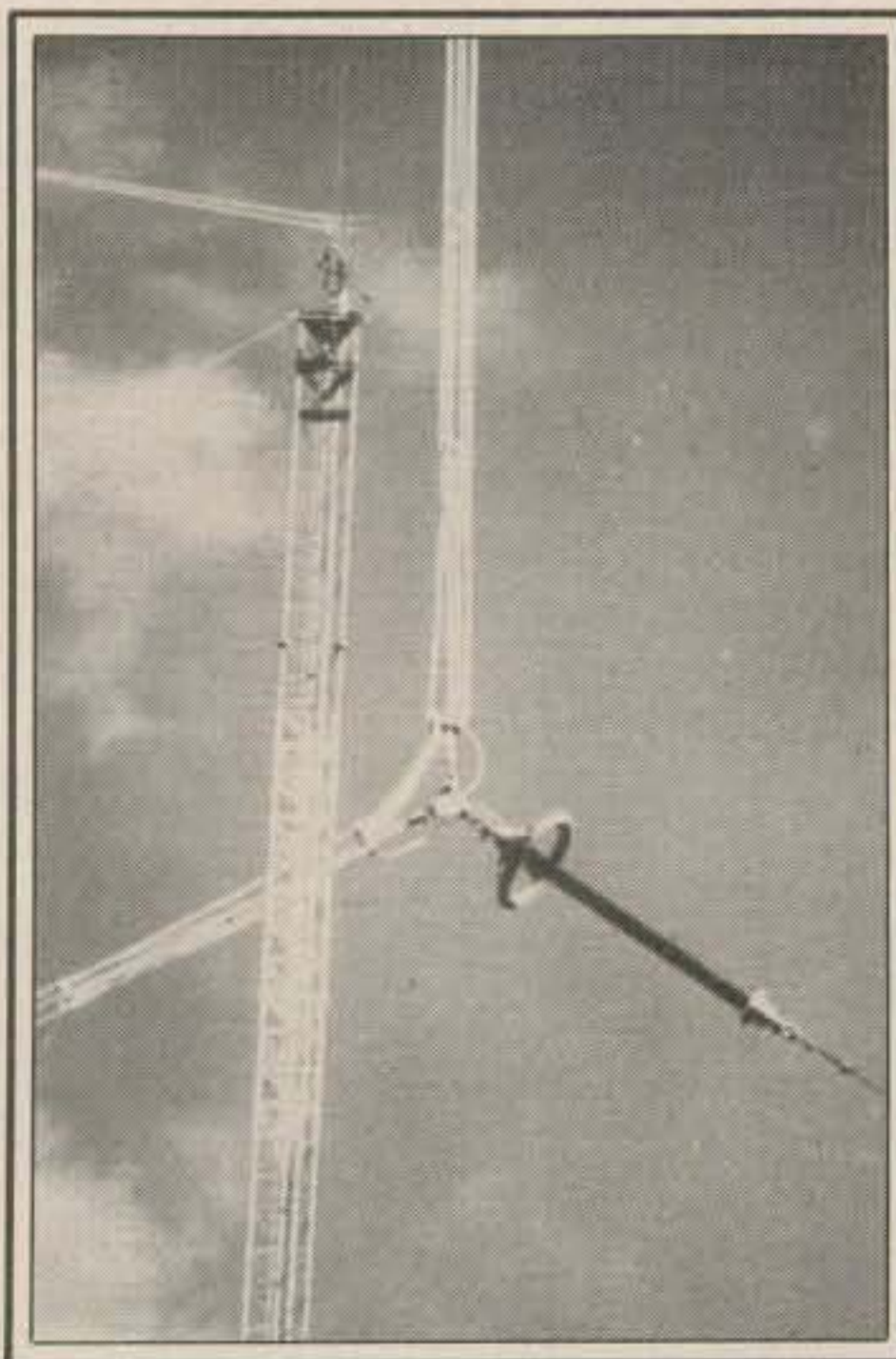
This photo shows the connection point between the WWVB/WWVL antenna downlead cage and the counterbalance insulator. The cage is comprised of six aluminum conductors mounted around rings approximately six inches in diameter. One of the support towers is also shown. (Photo courtesy NBS)
