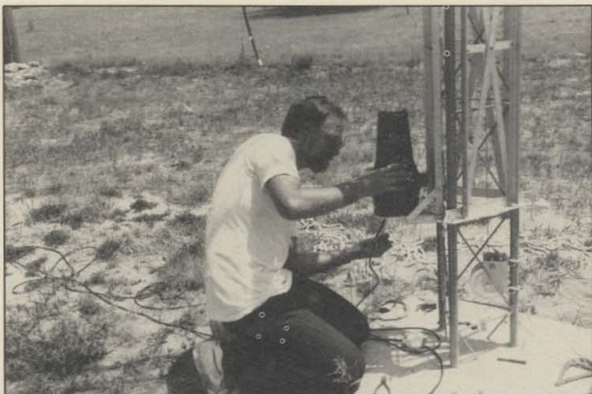
Photo F. K0JW shown mounting the rotor onto the Hazer working at ground level.
