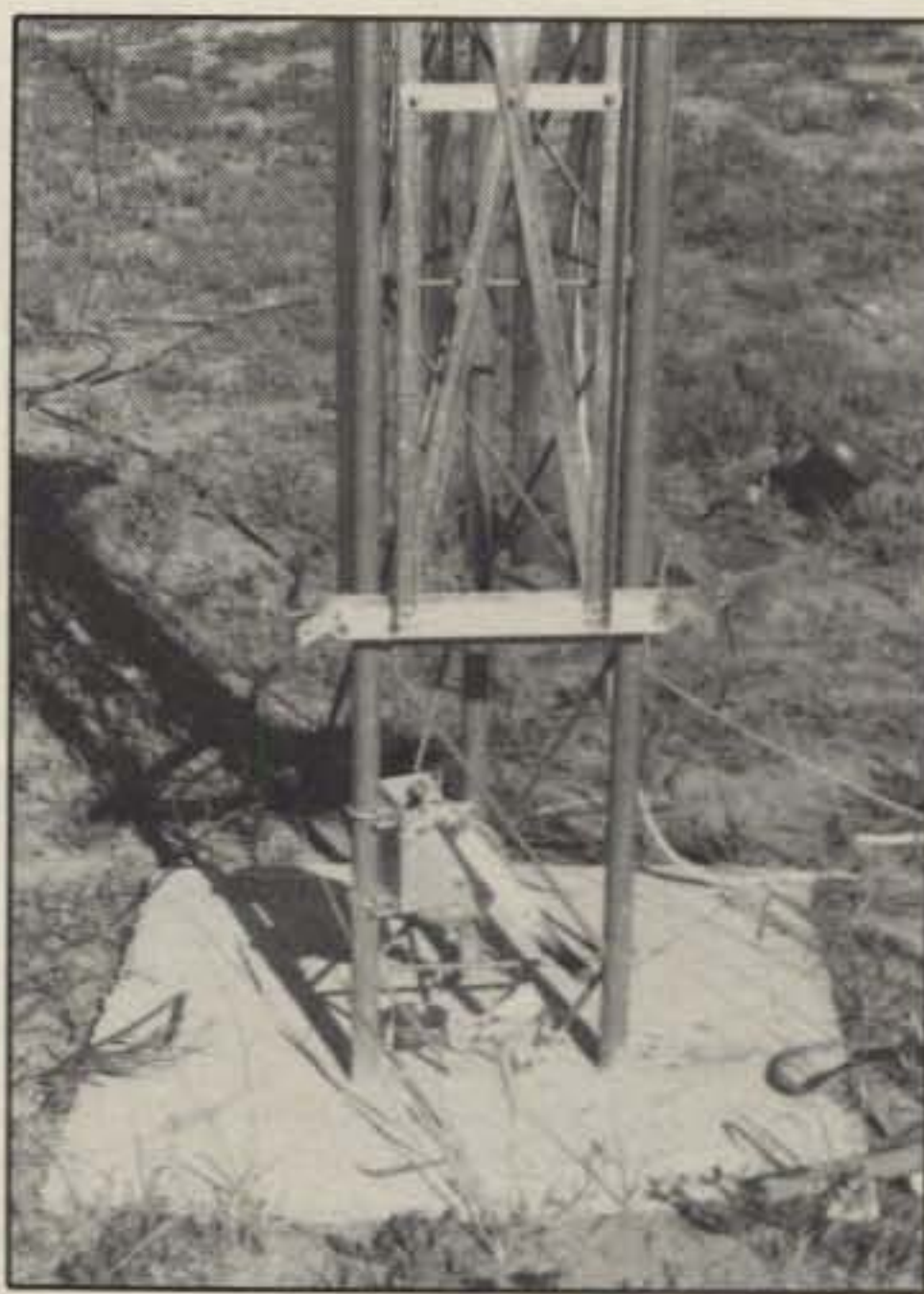
Photo E. The winch shown mounted at the lowest point on the tower to allow the Hazer to lower close to the ground.
