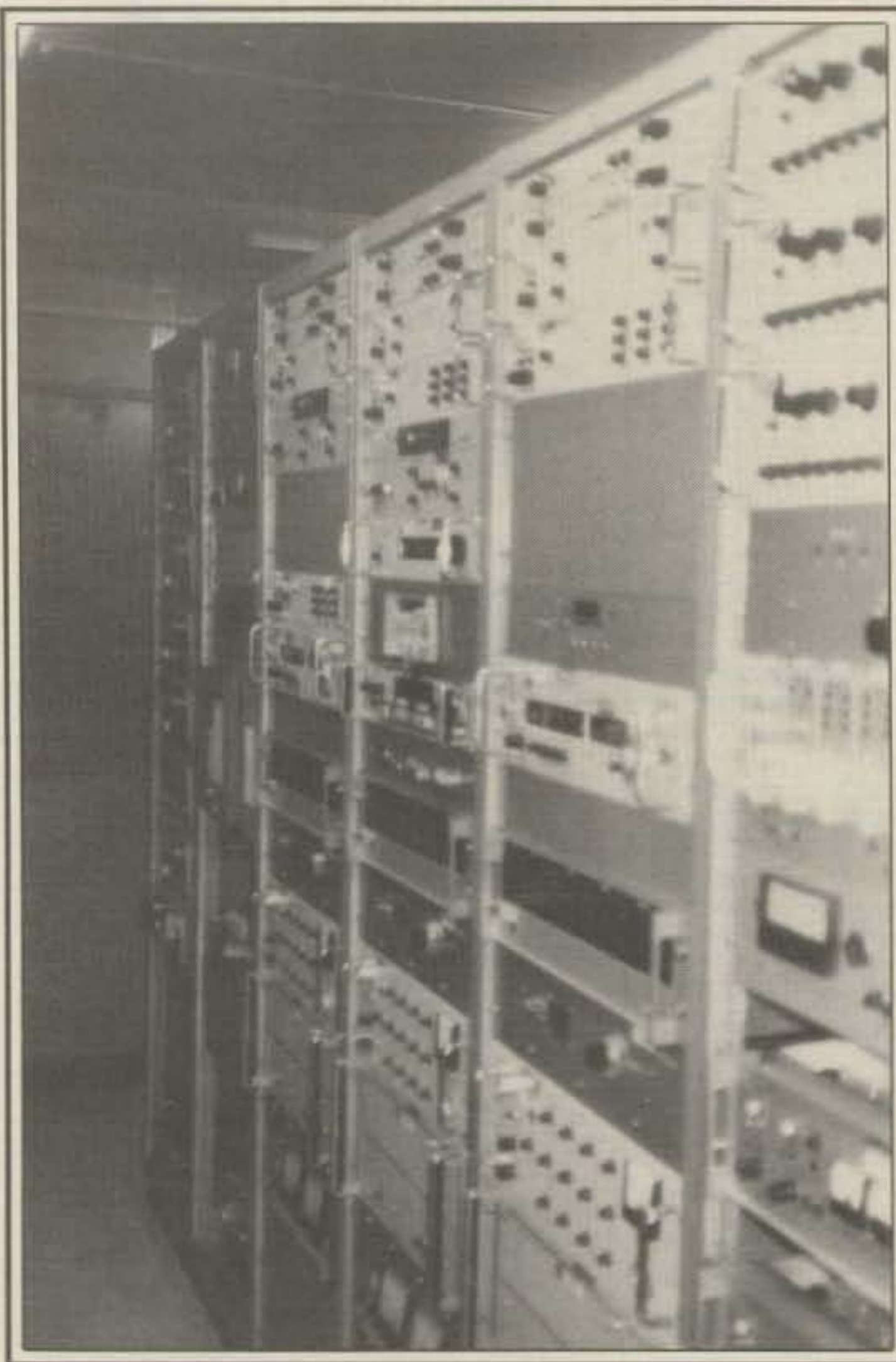
This is the array of control panels for time standards, frequency standards, and so on—lots and lots of buttons and controls.
