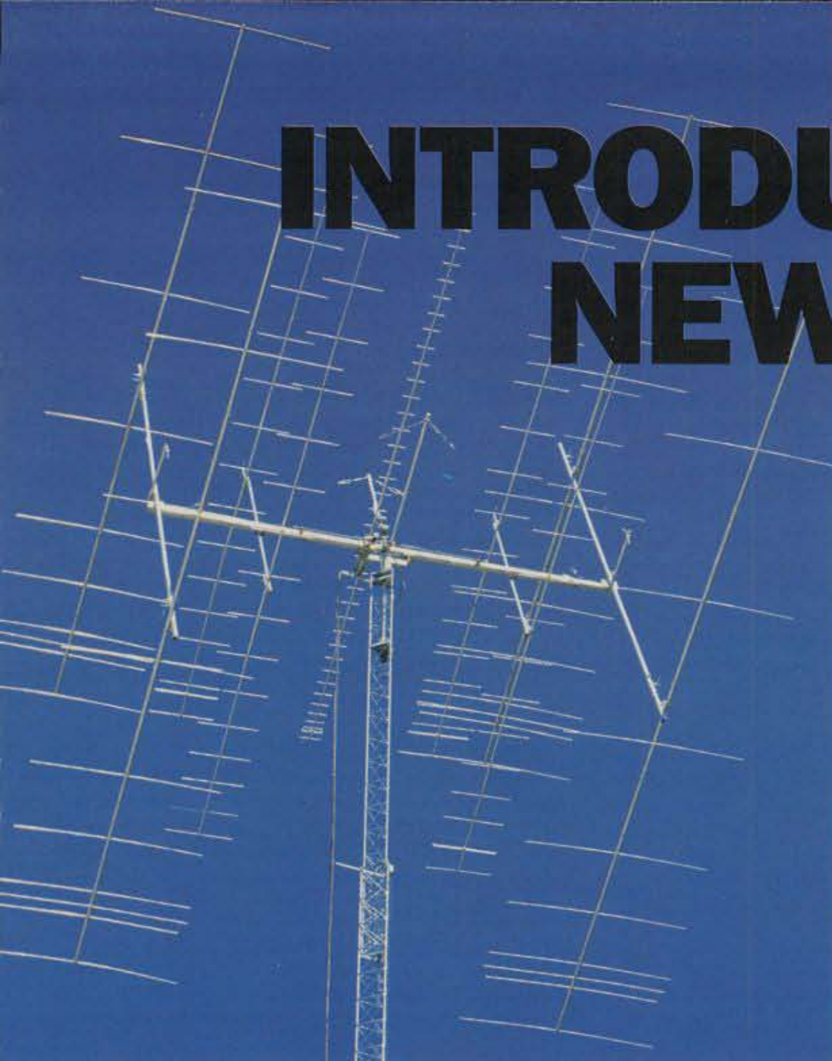
6-meter and 2-meter moonbounce installation. Four 6M-2WL, four 2M-5WL and one 432-13WL antennas in array on self-supporting 89-foot US tower at N7ML.
