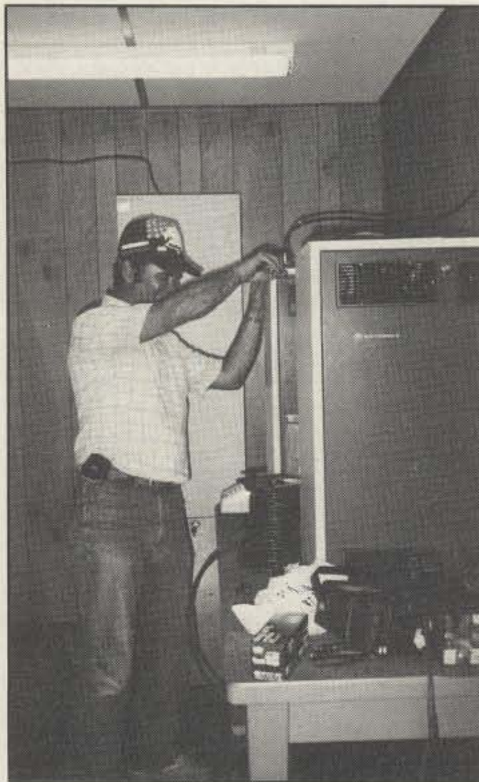
Rick, KK4DM, putting the coax to the new node transceiver at ABT10.
