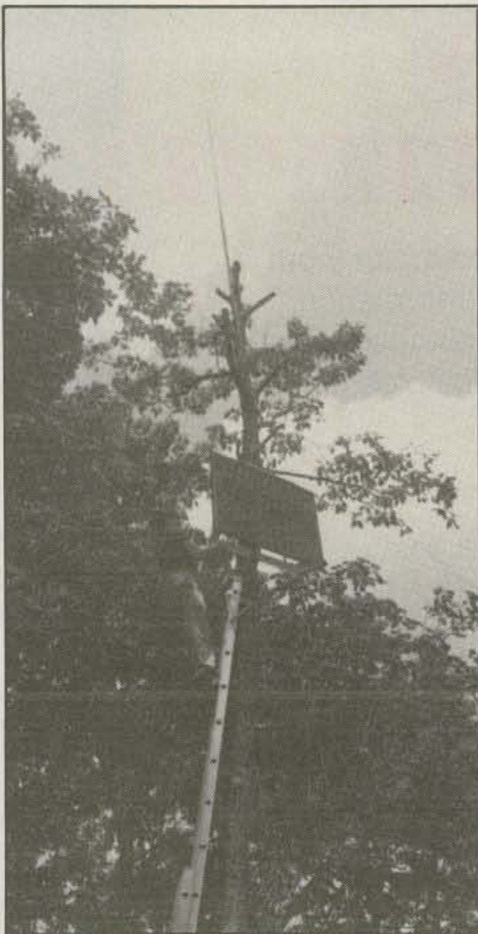
Photo 3- The solar panels mounted so they will receive optimum sunlight.
