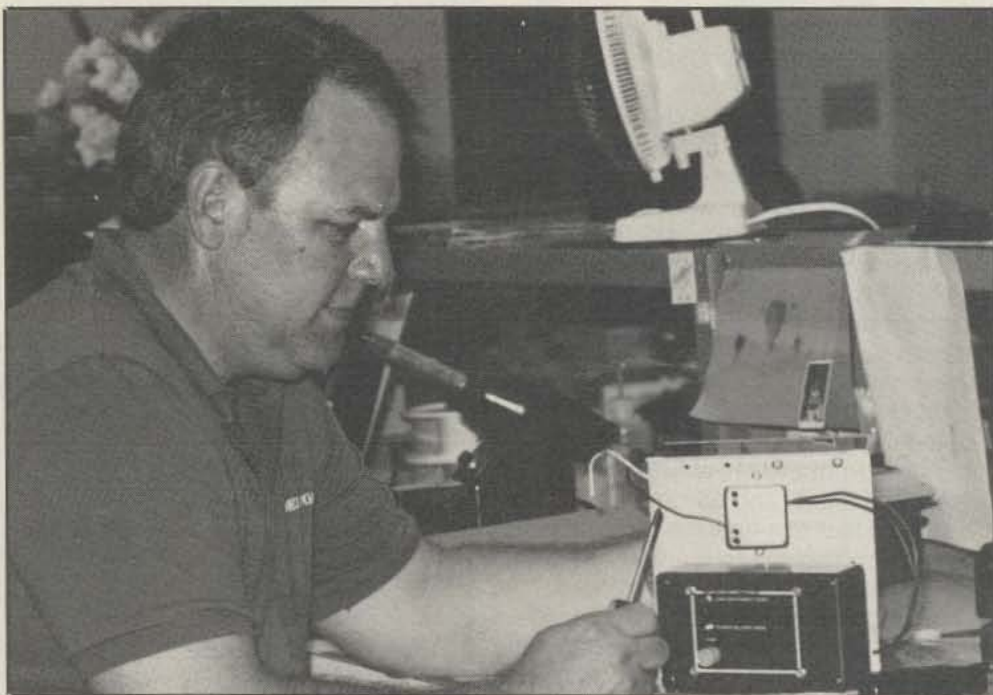
Photo A— Near the top of the panel is the M8 Sun Selector charge controller.
