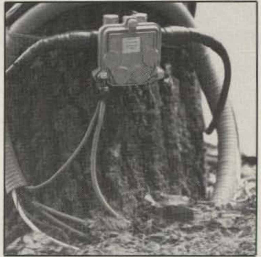
Photo D- The Cable Innovations Lightning Protector used in the project.
