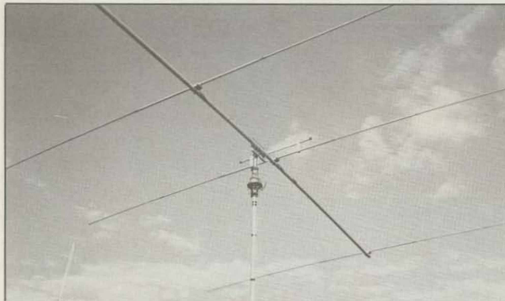
Here is one shot of the installed beam. The feed line is run from the boom to mast mount, and then down the support pipe. This is the special gamma matching assembly. The coax feed is brought up inside the mast, from the boom to mast mount, and then fed up through the gamma.
