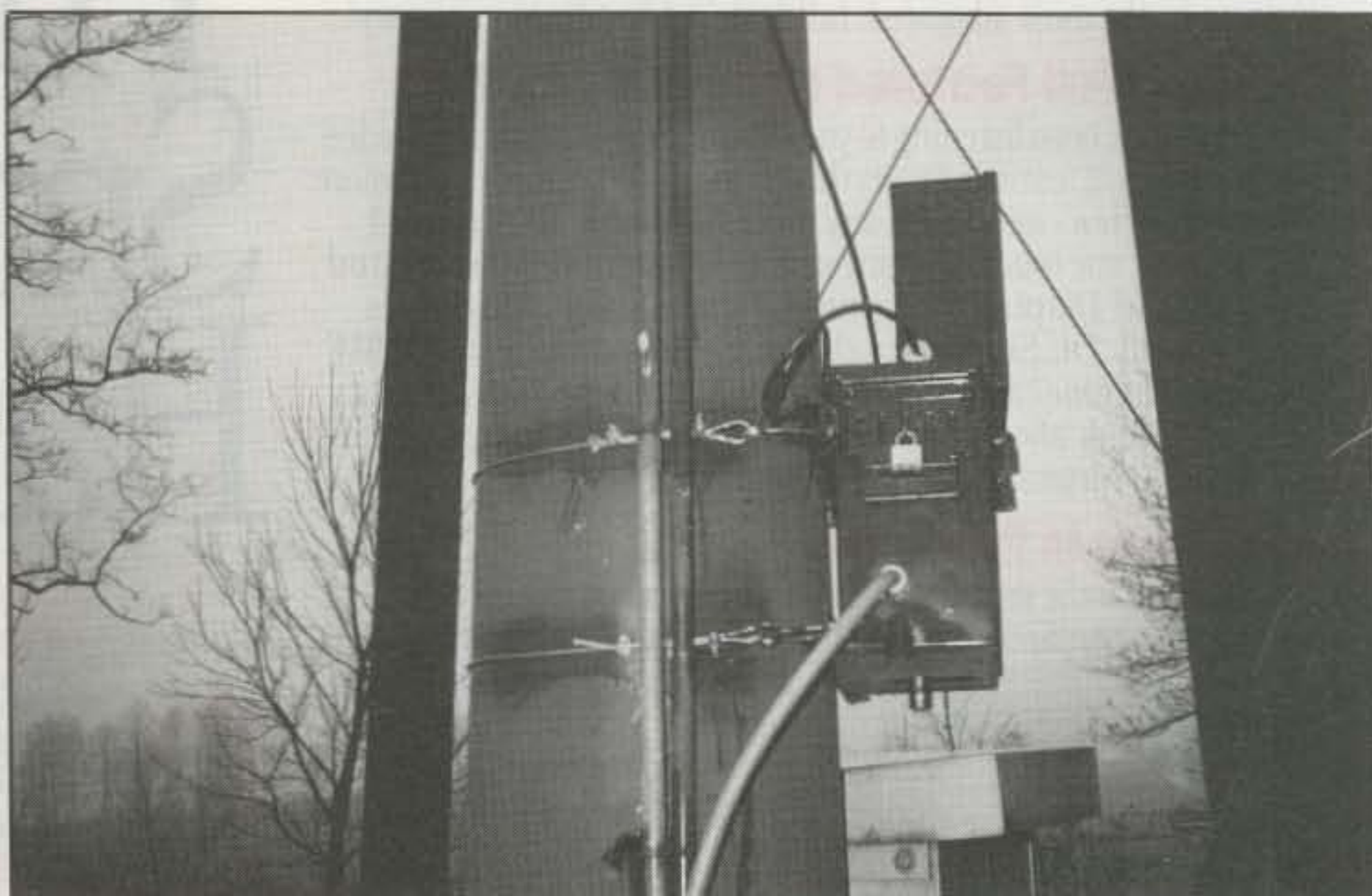
Photo 5— To prevent oxidation from rain water, a heavy compound was used on the water tank leg where the unit was attached to the water tank supports.
