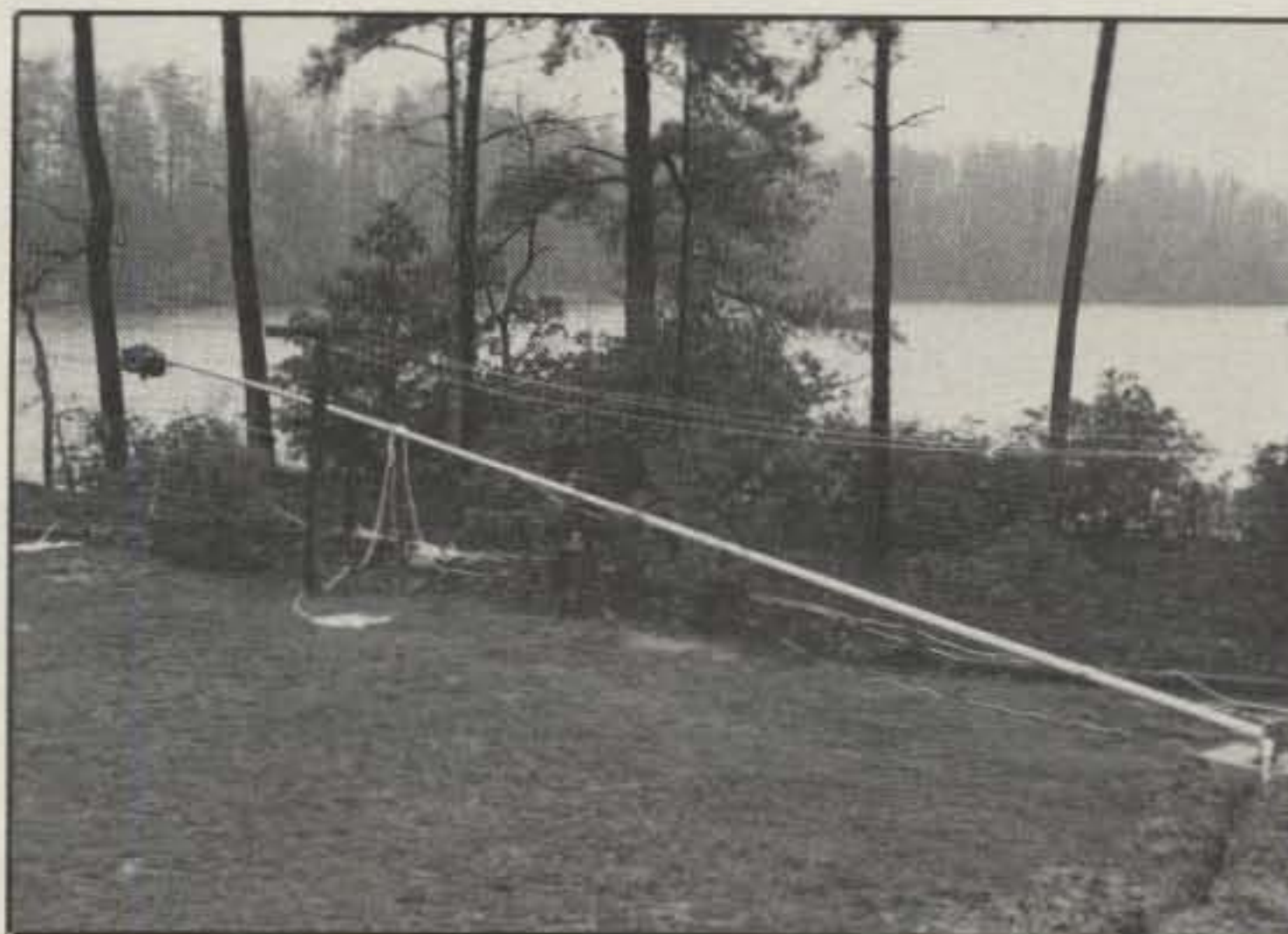
With the project completed and guy lines attached, the antenna is ready for raising.
