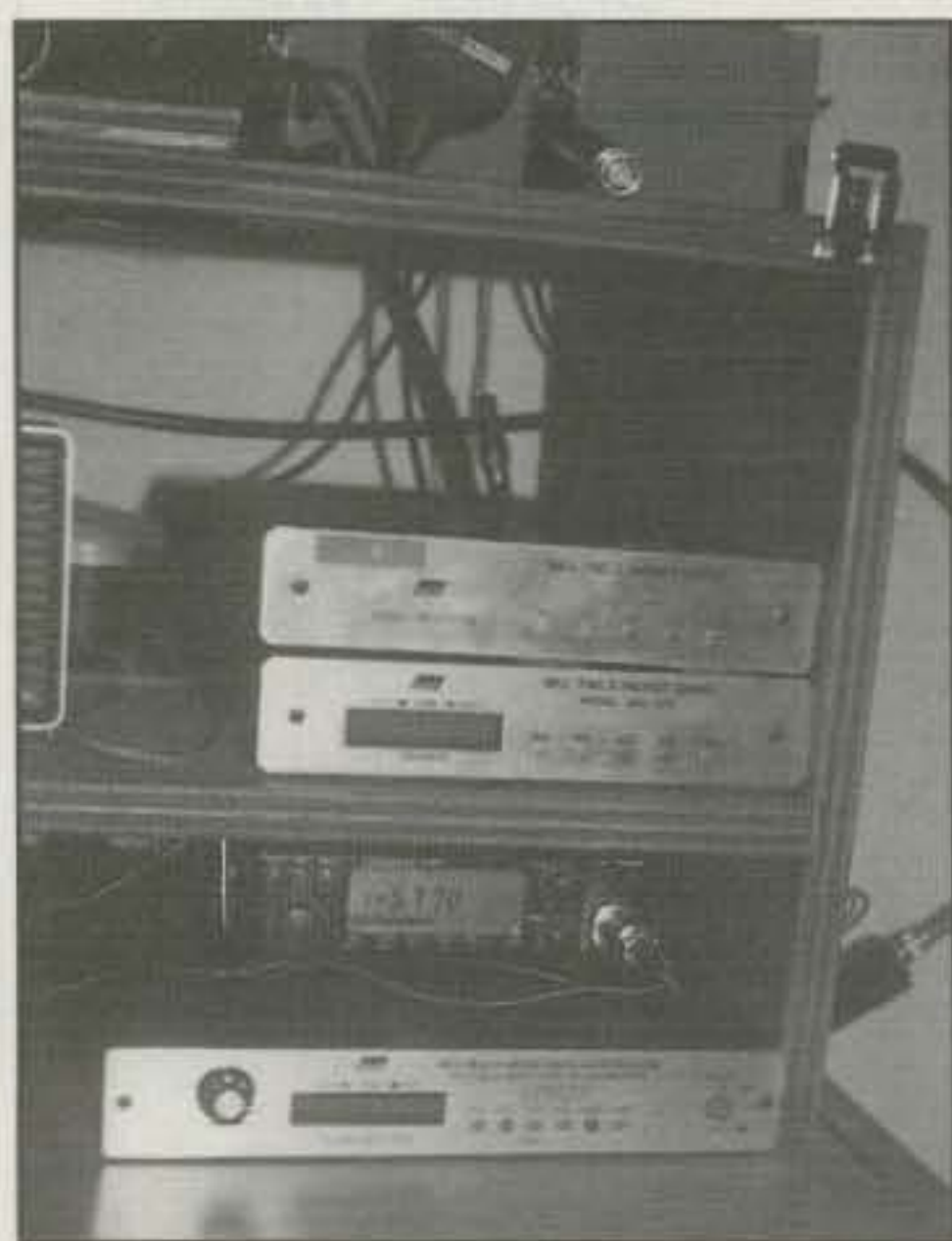
SEDAN X1J2 node of Chuck Beckham, N4XZV. Chuck is SYSOP of N4XZV-7/CGA at Conyers, Georgia. N4XZV-7 is fully supported with a pair of 100 ampere "Dynasty" maintenance-free batteries. The battery bank is kept alive by an ARCO 16-2000 solar panel array.
