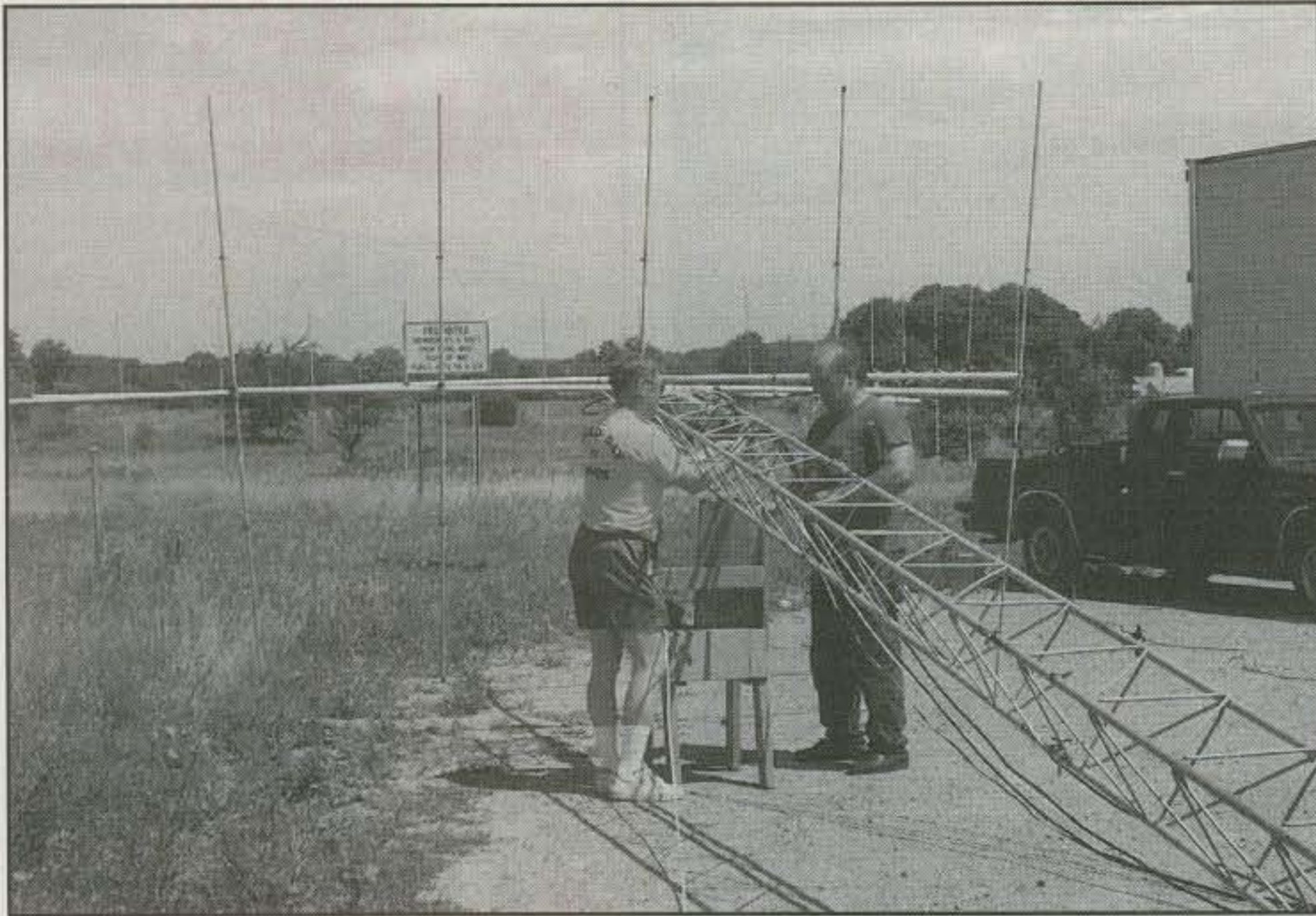
Dave Bostedor, N8NQS, and Dave Hogston, KB8MXX, install the 6 meter antenna at one of their Rover stops. (Photo courtesy N8NQS)
