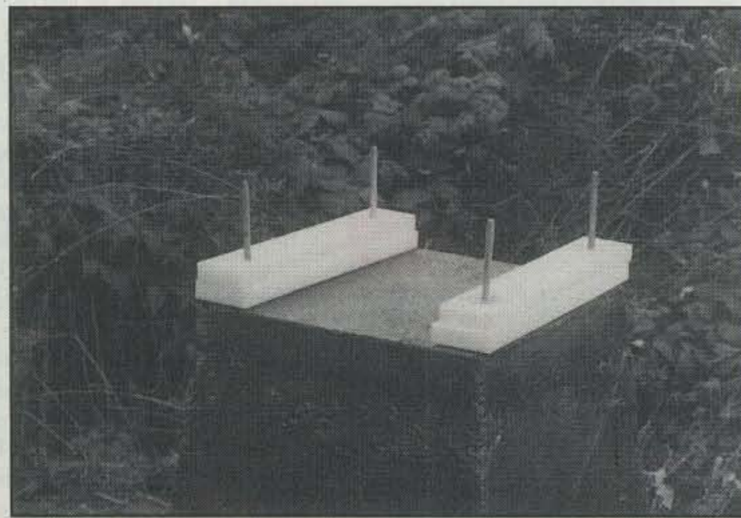
Here we introduce the first stage in insulating the tower from the concrete base. The two strips of 1 inch thick Tivar 100 can be seen on opposite sides of the concrete base.
