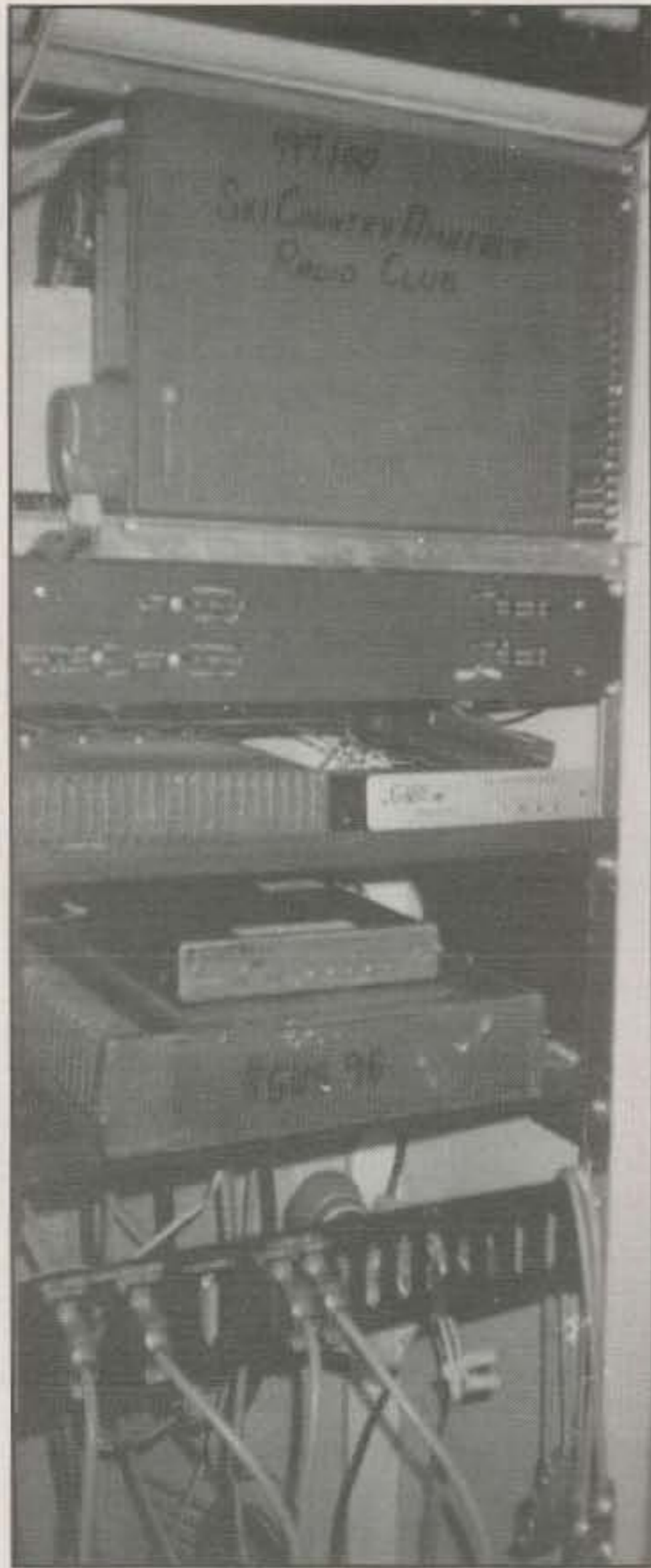
Photo F- NØMOR's installation includes a 447.1 repeater, 447.1 controller, KØGUZ-1 1200 baud port at 145.010 MHz, KØGUZ-2 441.050 backbone 9600 baud, and diode matrix for other nodes in the stack.
