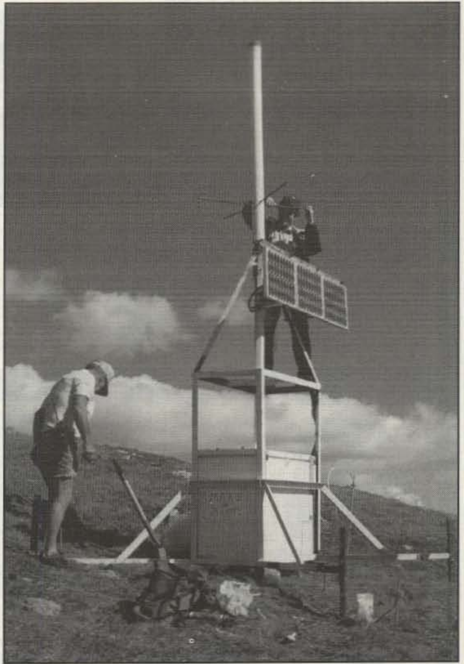
Taking advantage of the nice weather in September 1993, VE7HRC and VE7EMS quickly secure the module to the mountain and set up the antennas.
