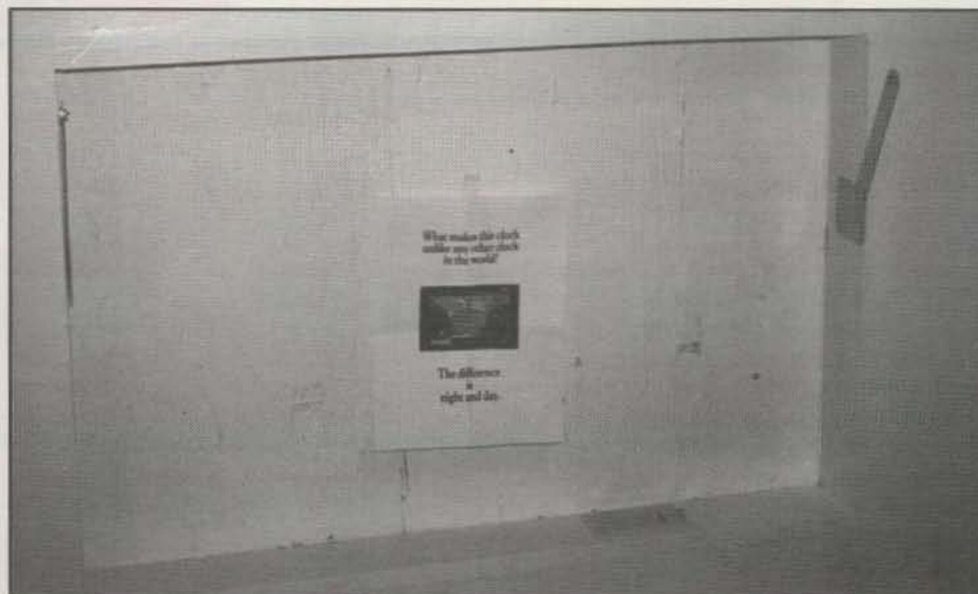
A few days later the hole is complete, the wall is clean and shiny with fresh paint, and the brackets and outlet are in place.
