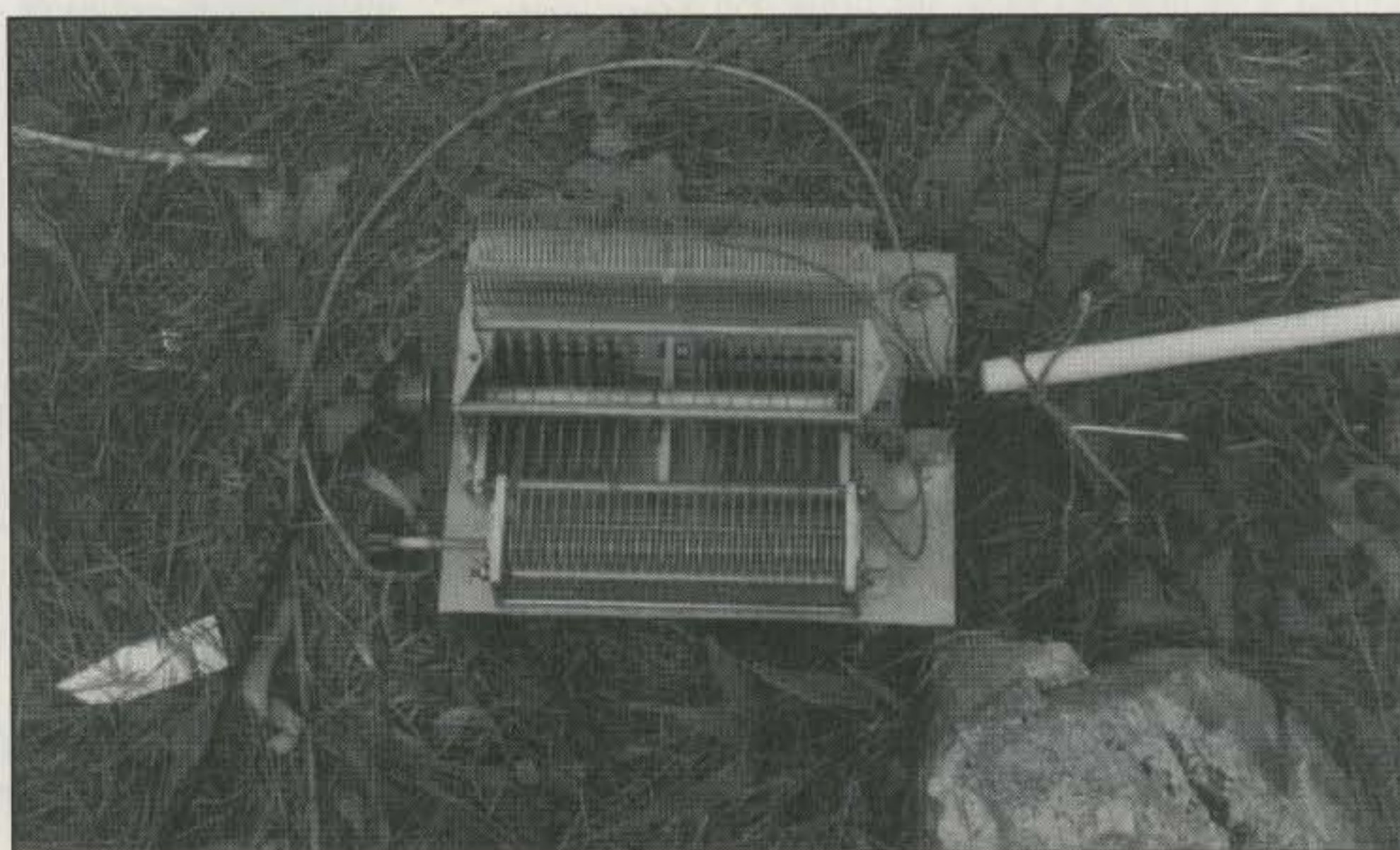
The coil, capacitor, and relay are mounted on an aluminum plate. The tuning unit sits off the ground on a few bricks to keep moisture out.
