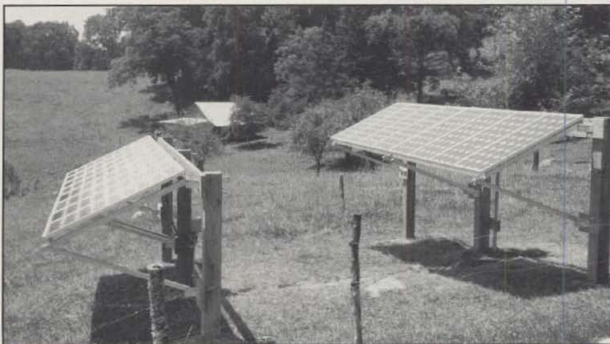
Photo 7— Solar panels are an excellent choice of low-maintenance and long-term alternate energy, especially when backed up with a generator for times of heavy loads. (Photo courtesy Tom Harrington and Universal Electronics, Inc.)
