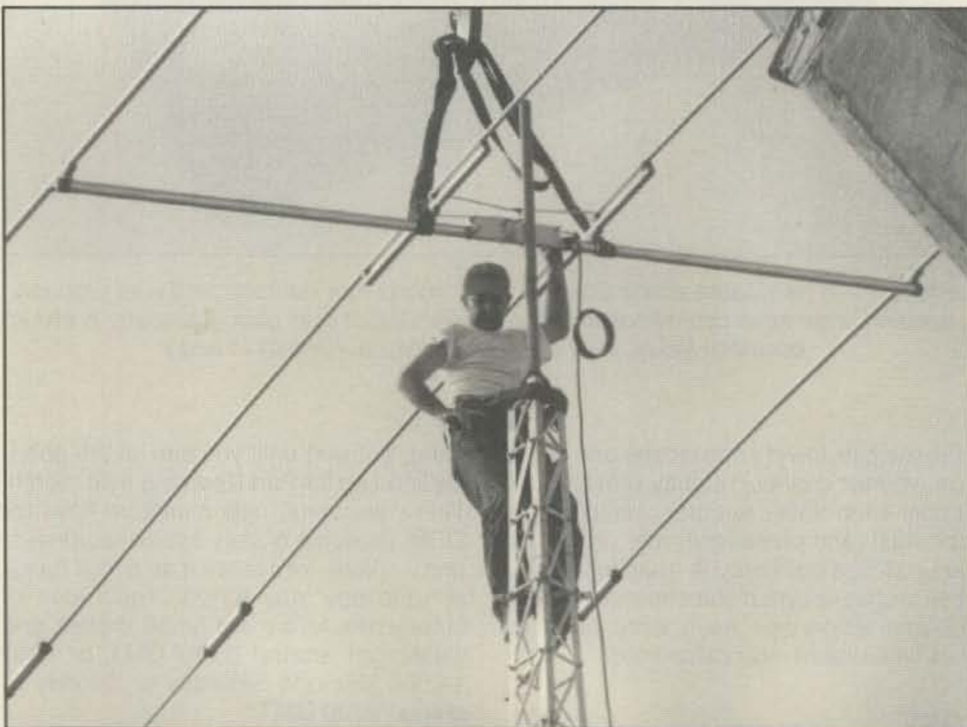
Jim, SV2CCA, bolts a four-element, five-band Mosley TA53M to SV2CWY's roof tower.
