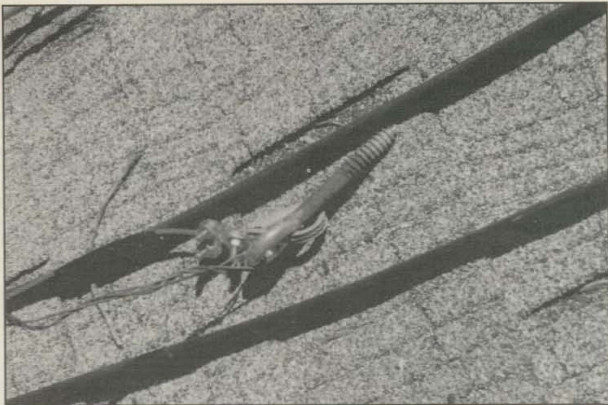
To bring the point home, the eyebolts all showed rust and discoloration on the part of the screw that was in the wood.
