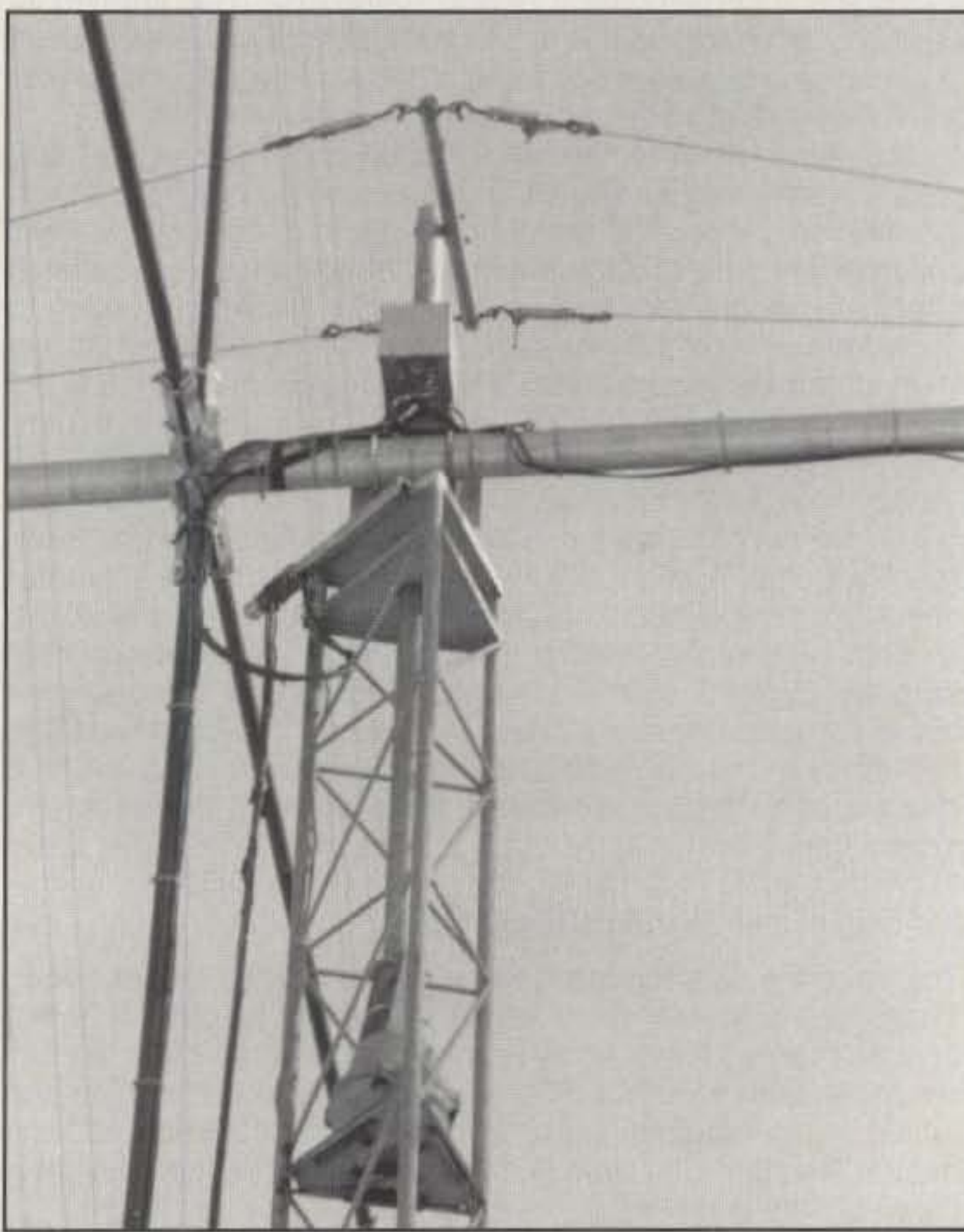
Boom support and turnbuckles for boom sag adjustment.
