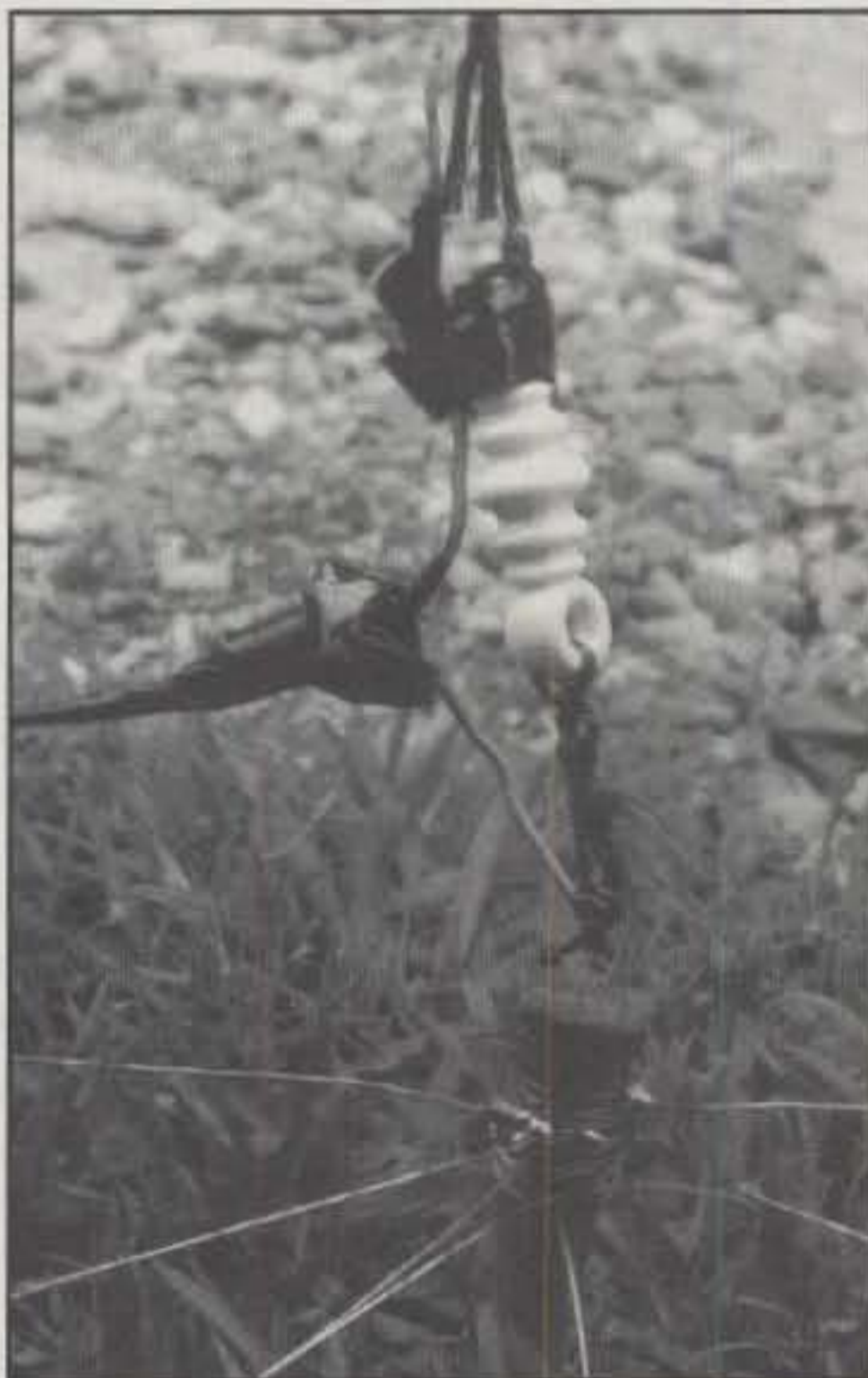
It's simple and most of all it works. This is the feed point of the 160 meter inverted-L antenna.
