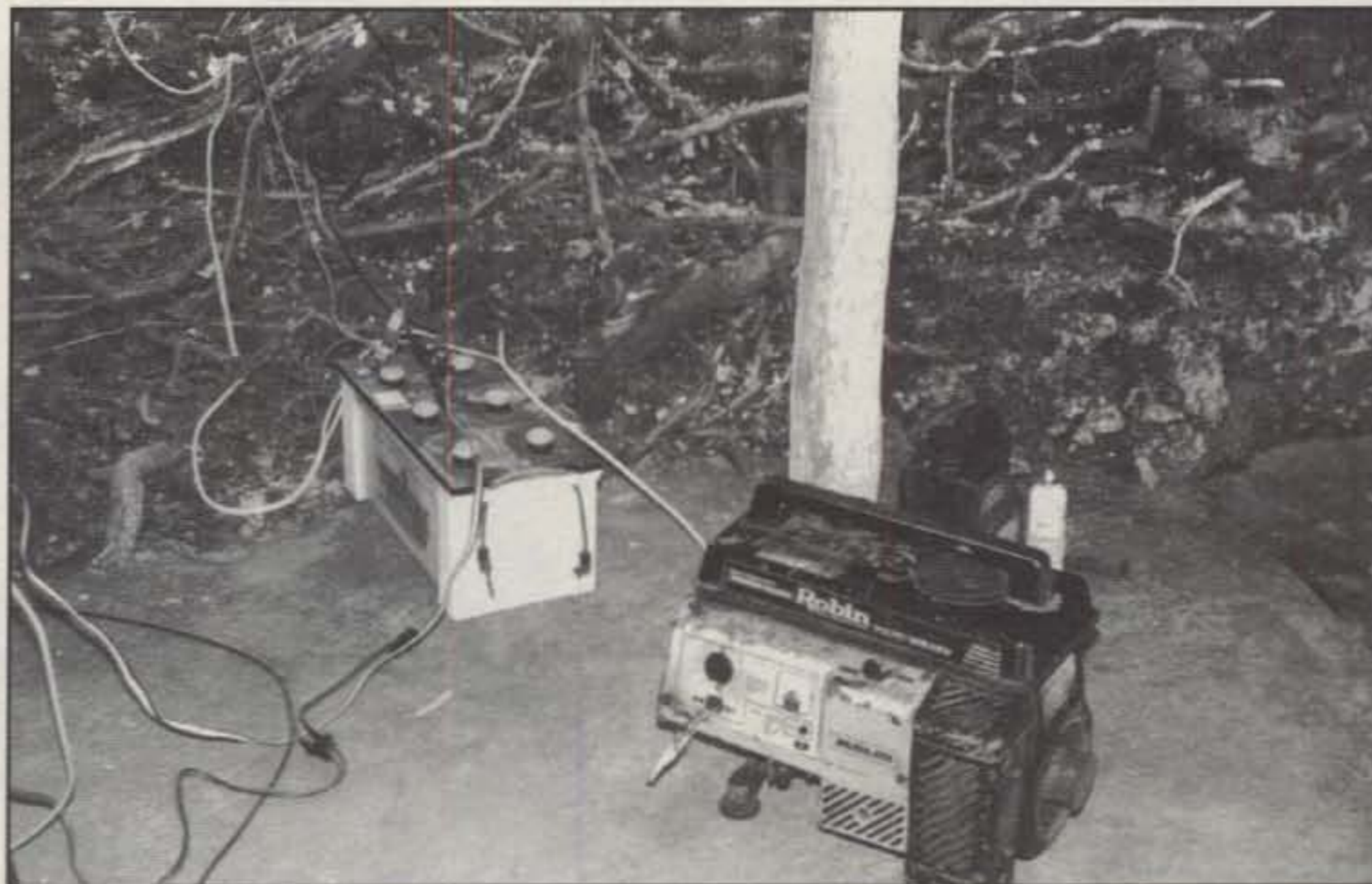
Temporary power: a battery, generator charging output, and solar panels.
