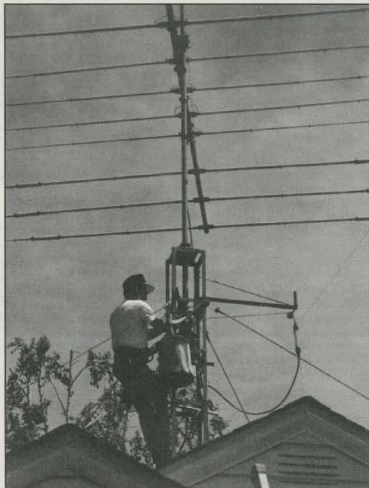
With any antenna project, remember: safety first. Always use a safety harness. (On the roof: Gary Woodhouse, K2UU.)
