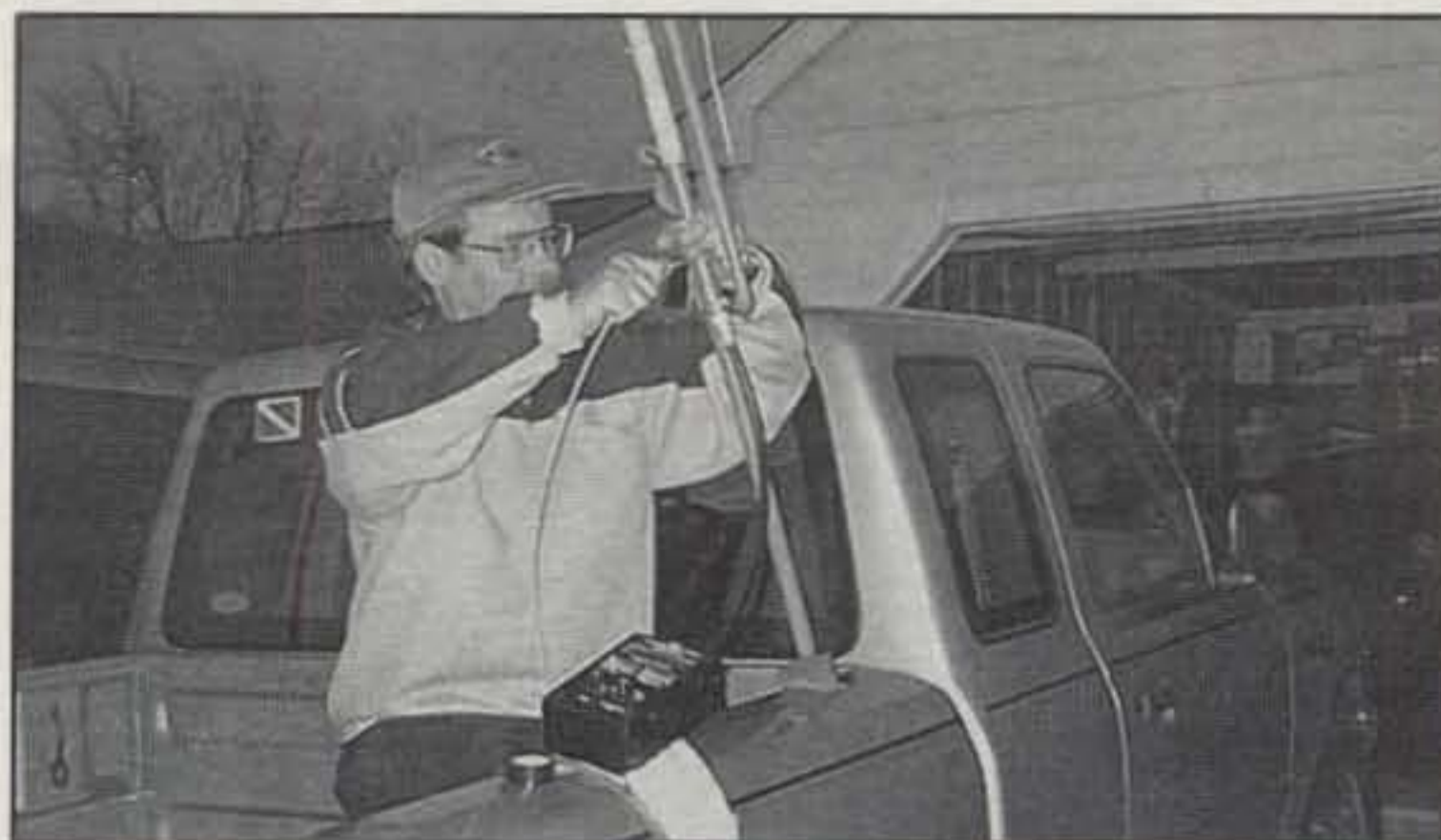
Photo 5— There is no "hard" connection from the feed-line center conductor to the copper pipe at all. It's inductively coupled. I mounted an SO-239 on the cross portion of the "J" as shown. [But Eddie, what about the built-in, DC ground lightning protection of the J-Pole?—K4ABT]
