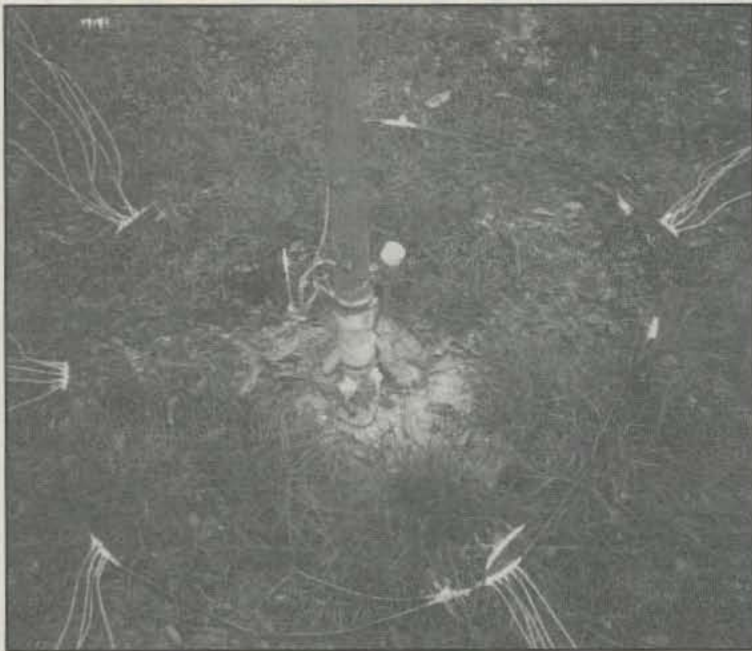
Photo 3— The ground system. The loop is connected to the buried ground conduit and 25 radials. The white material is liquid tape the author was testing for this application.
