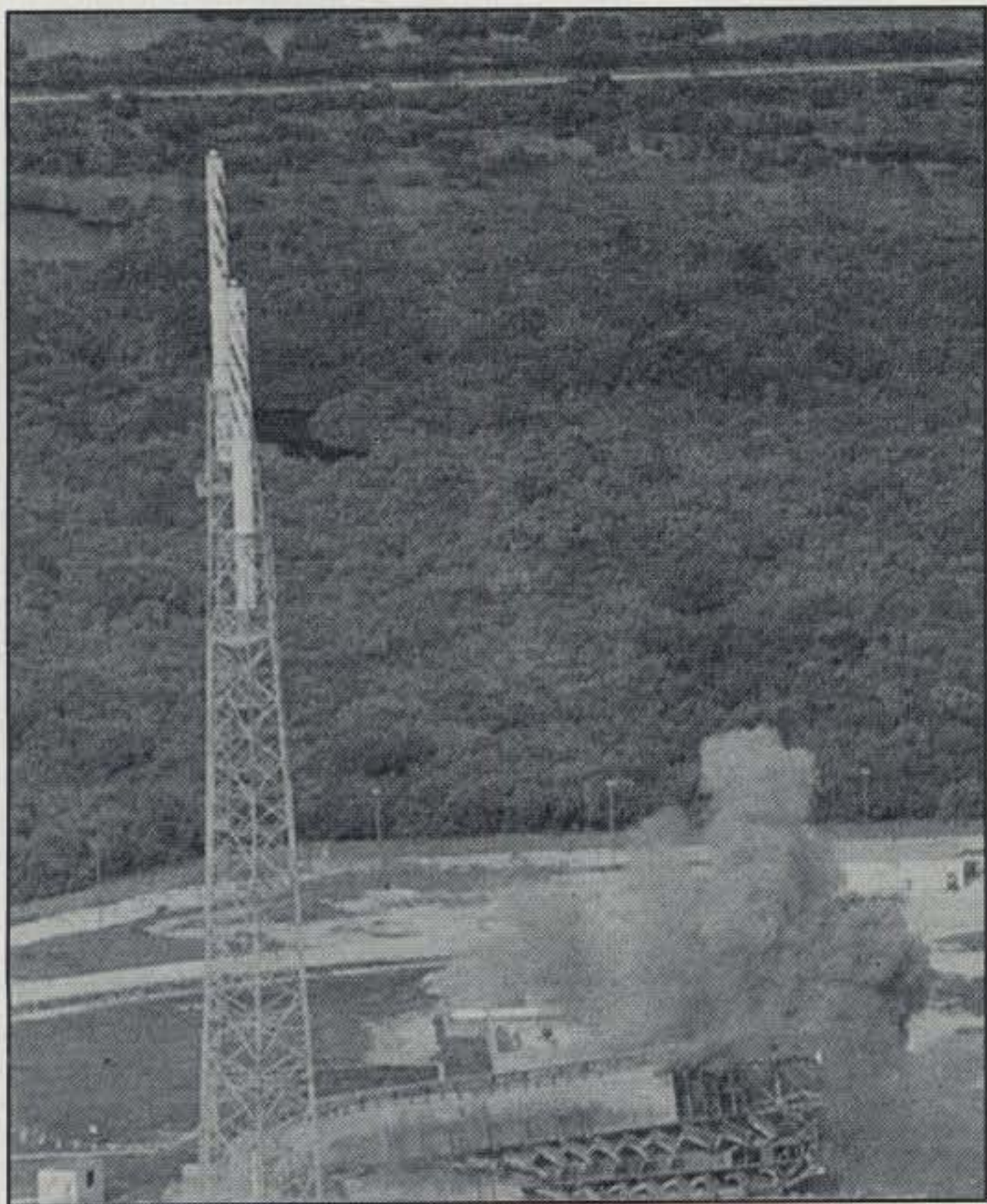
The 2 million pound Umbilical Tower (left) and 5 million pound Mobile Service Tower (right) at Launch Complex 41 are topped by explosives to make way for the new Atlas V launch vehicle. Among other satellites, LC-41 was used to launch Voyager, Viking, and OSCAR 4—the first high-altitude amateur radio satellite. (NASA photo)
