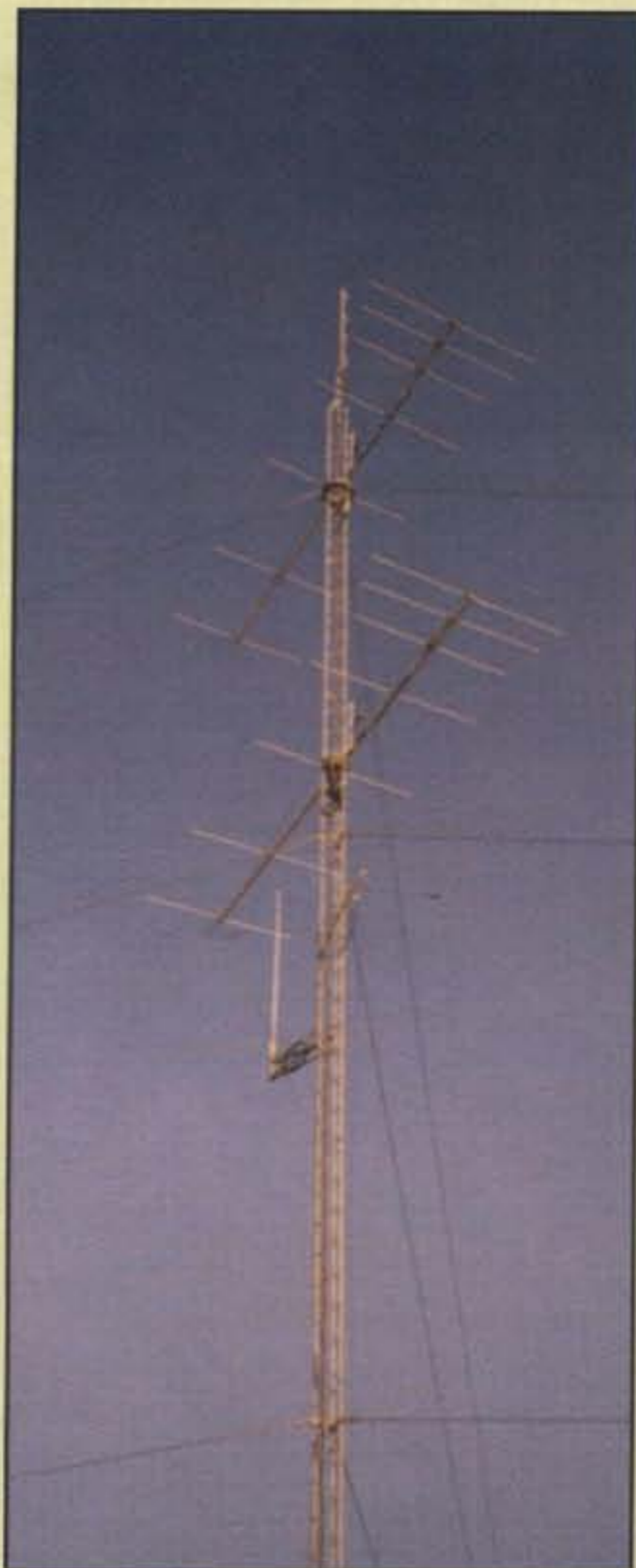
Photo 7— Job complete. The rotating section turns two 7-element, 6 meter beams installed at 61 and 83 feet, respectively. As you can see, it's very important to plan your installation so that the lower Yagi can turn freely between the top two sets of guy lines. The antenna below the rotating section is a half-wave vertical for 6 meter FM.
