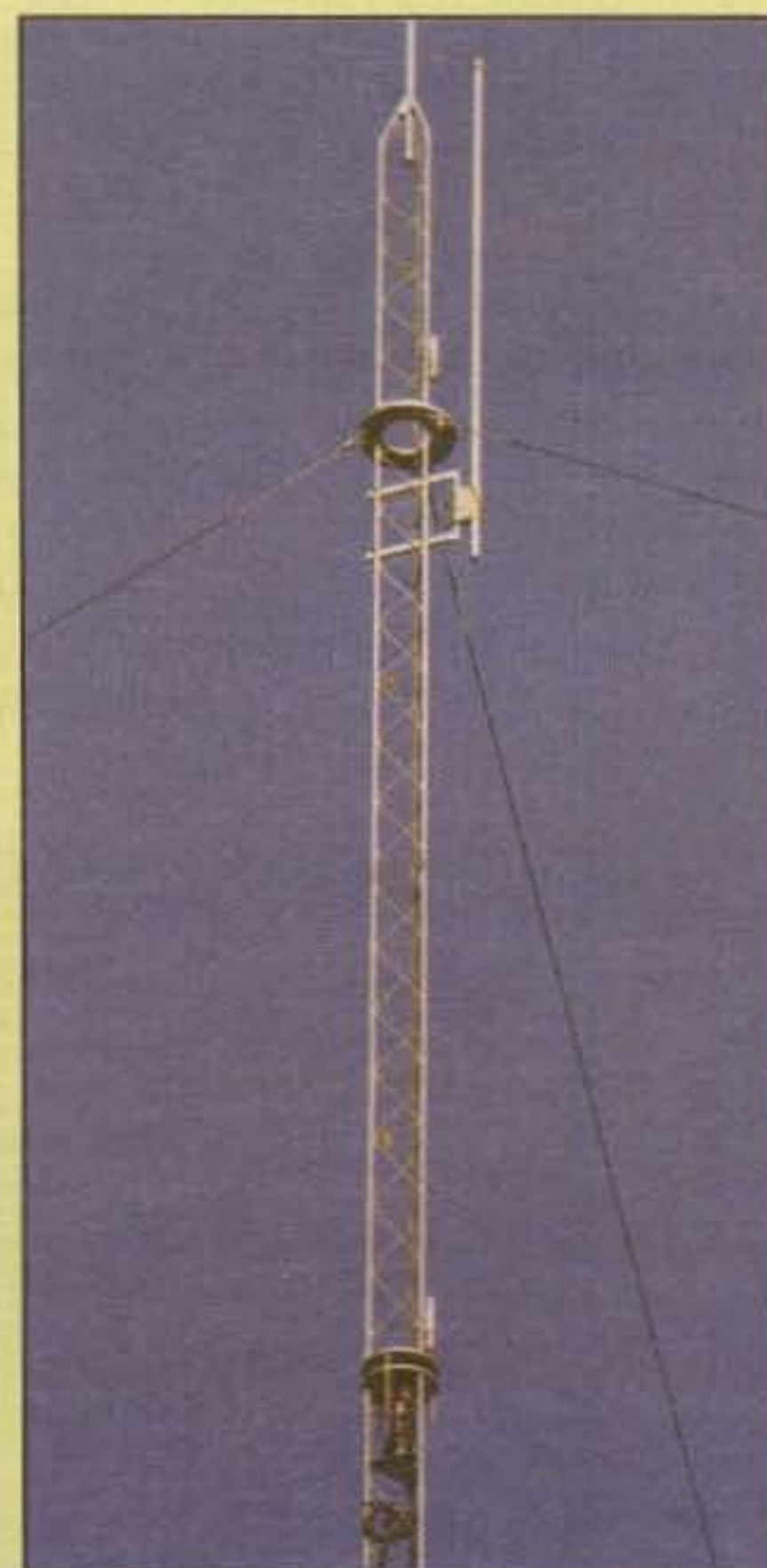
Photo 6— The rotating section of the author's tower. Working up from the bottom of the photo, you have the rotator and main bearing, the rotatable tower sections, the guy ring, and the gin pole and adapter.
