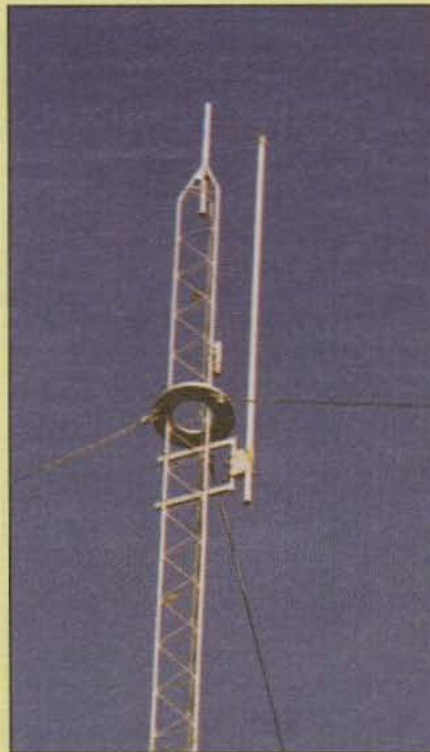
Photo 5— Upper portion of the tower seen with the guy ring installed and gin-pole adapter attached.
