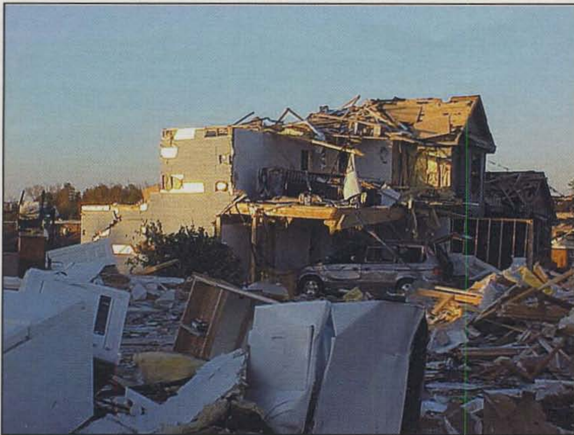
Hams reported major structural damage in several areas of the city. (Photo courtesy the National Weather Service)
