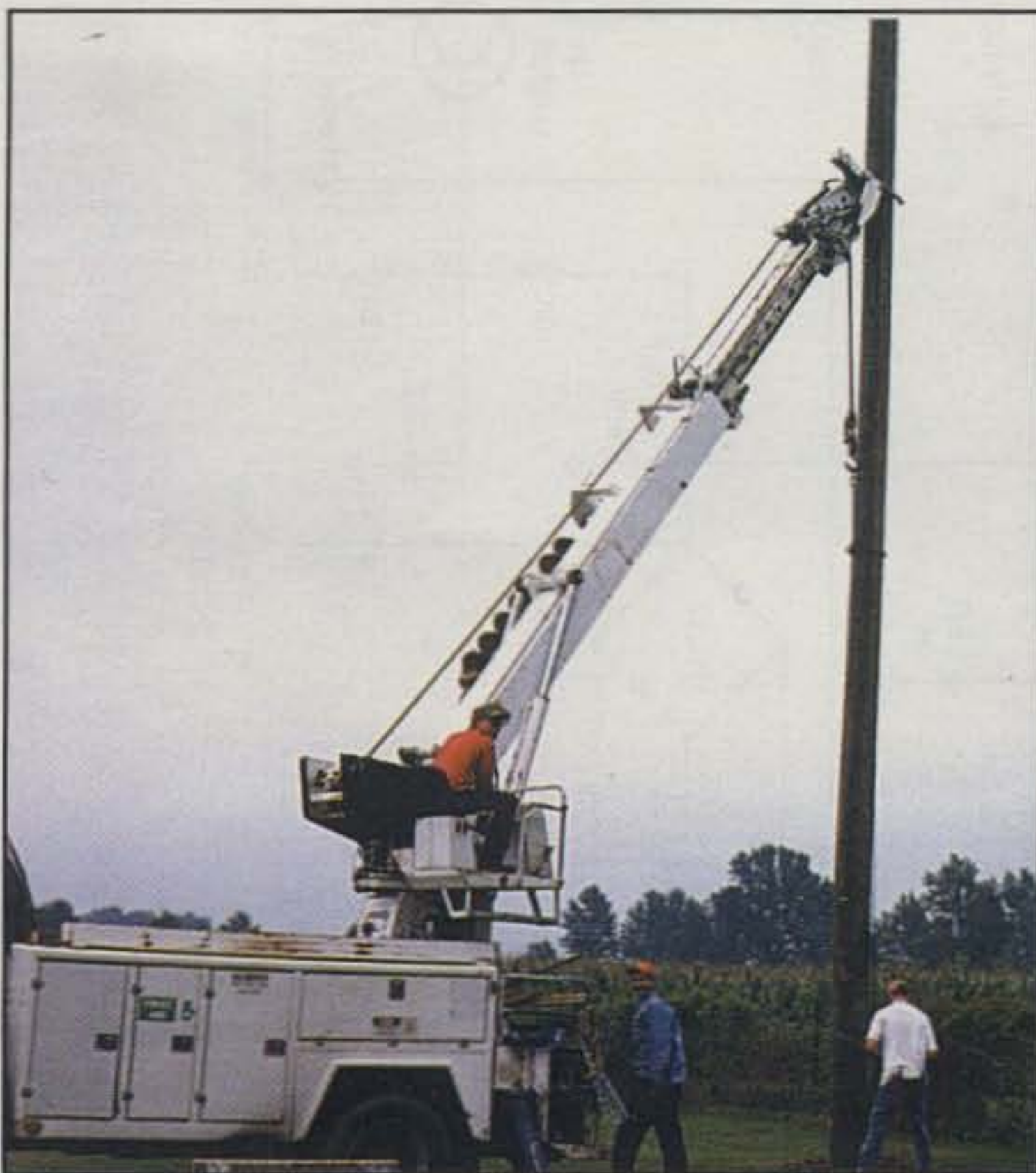
How do you put up poles like these? Well, you don't do it alone, that's for sure! Some mechanized help is a good idea, too. For ease of later construction, the pulleys were attached to the eyebolts before the poles were installed.
