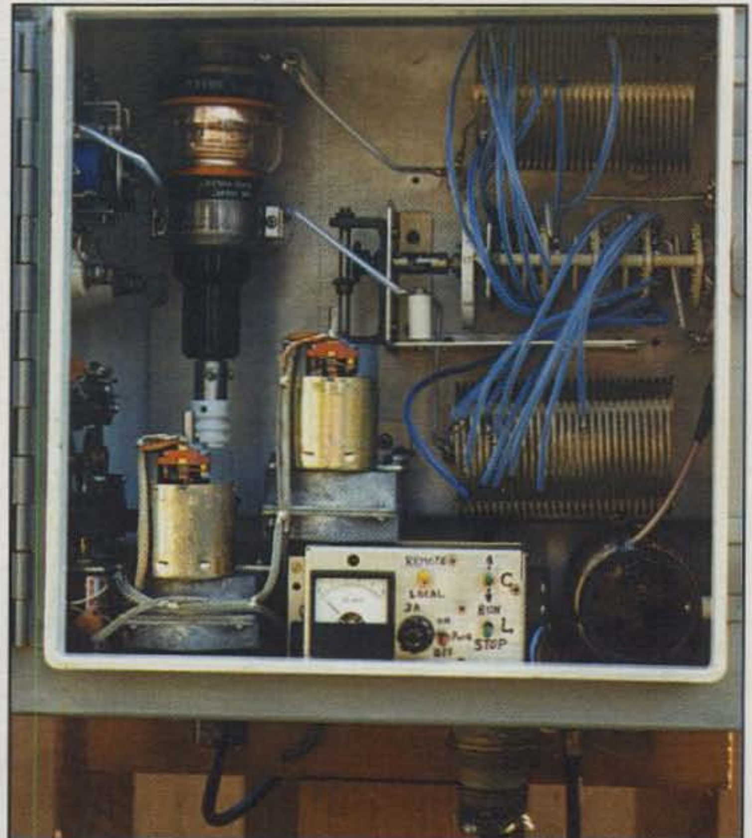
Interior view of the tuner box. Note that the tuner is outside, at the antenna feedpoint, so a weatherproof box must be used, along with grounding precautions.
