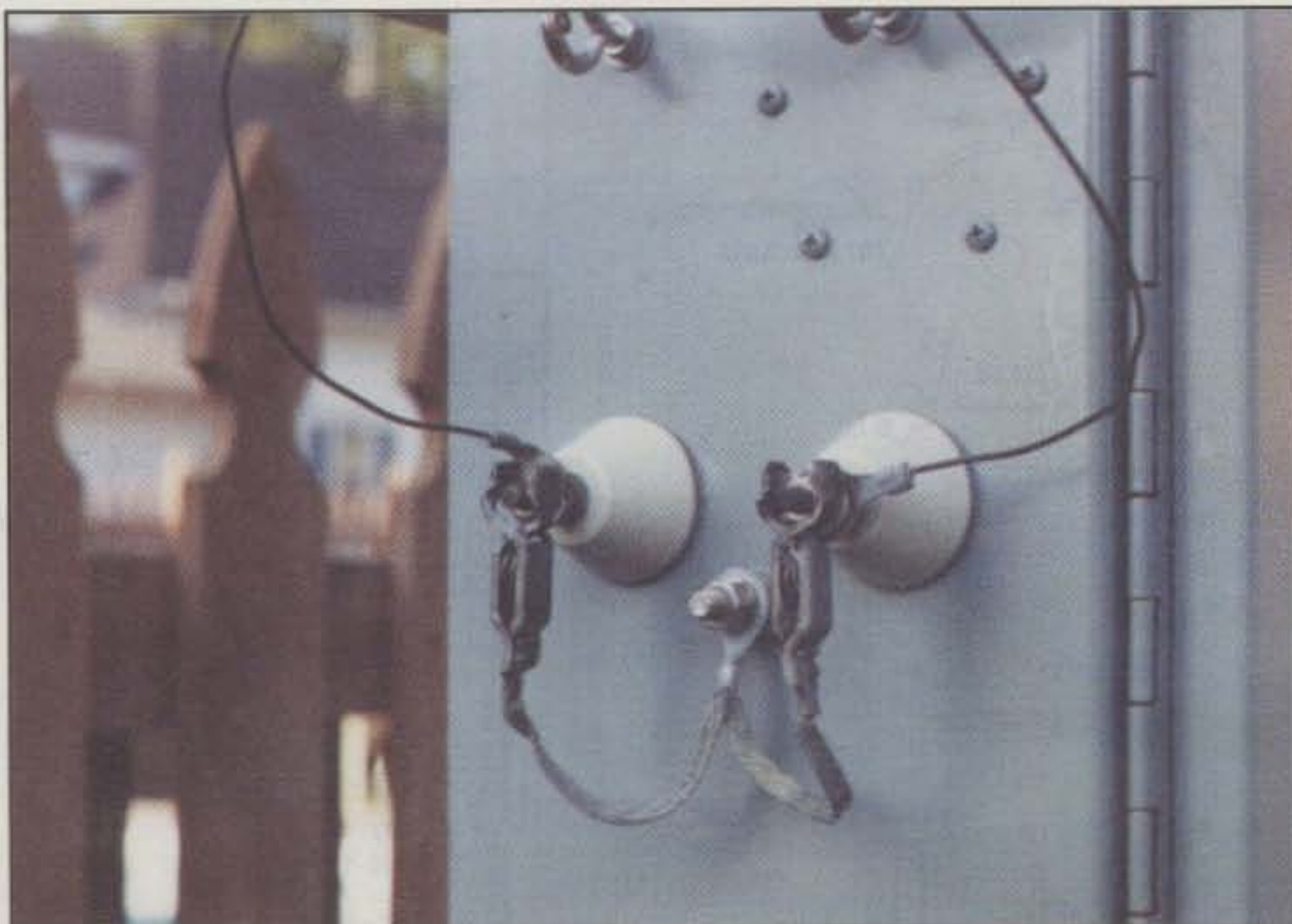
Grounding clips and strap attach to ground wire inside tuner box for manually grounding the antenna when a storm is approaching. An internal relay also grounds the antenna in the "off" position.
