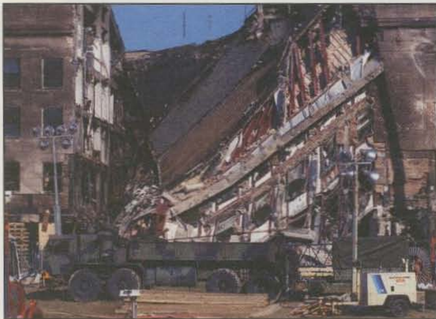
Damage to the Pentagon extended far beyond this section of the building, which collapsed after being struck by a hijacked airliner. (US Dept. of Defense photo by R.D. Ward)
