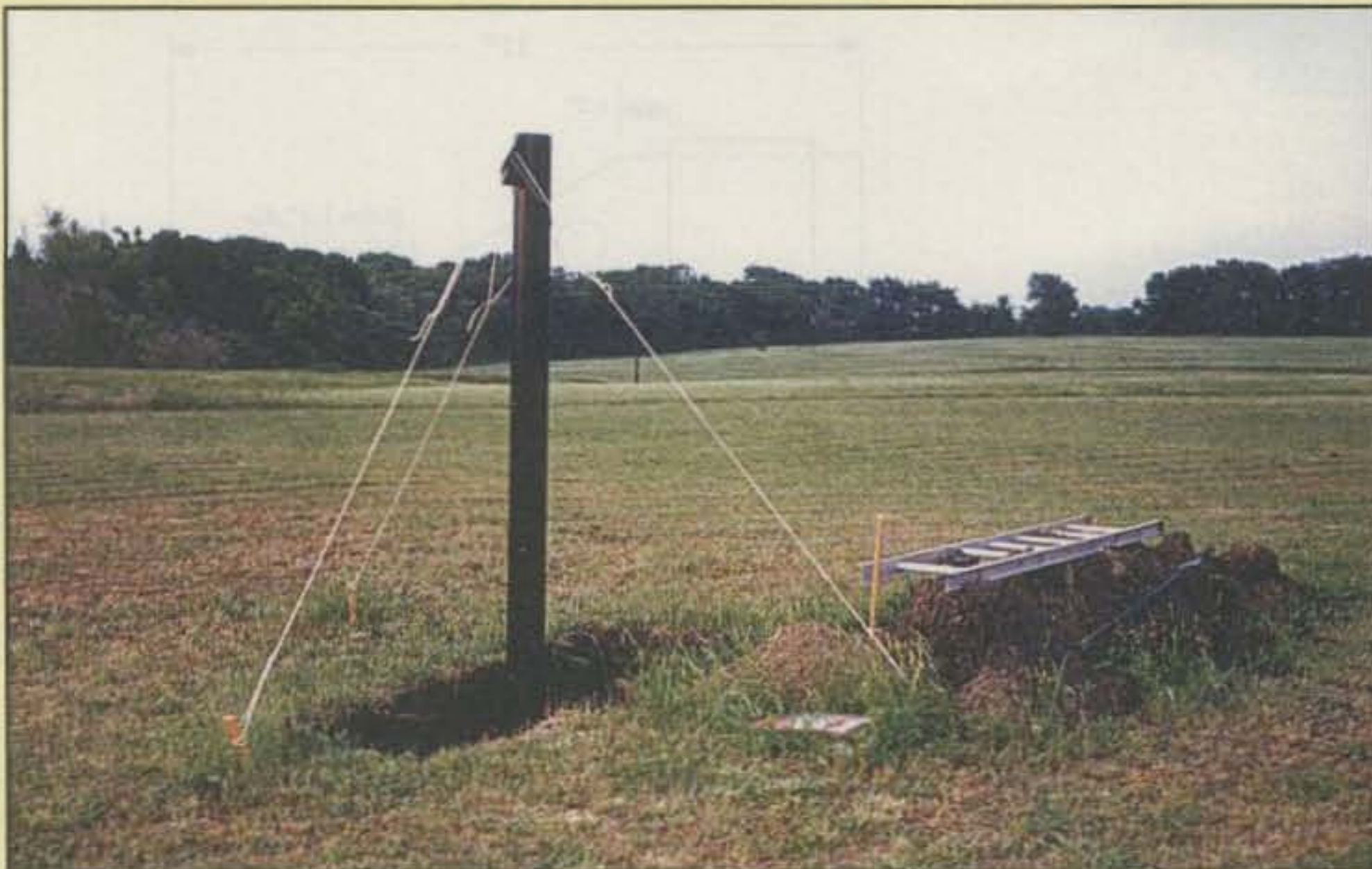
Photo D— The three temporary guy ropes are shown here keeping the pole steady so the concrete can be poured.
