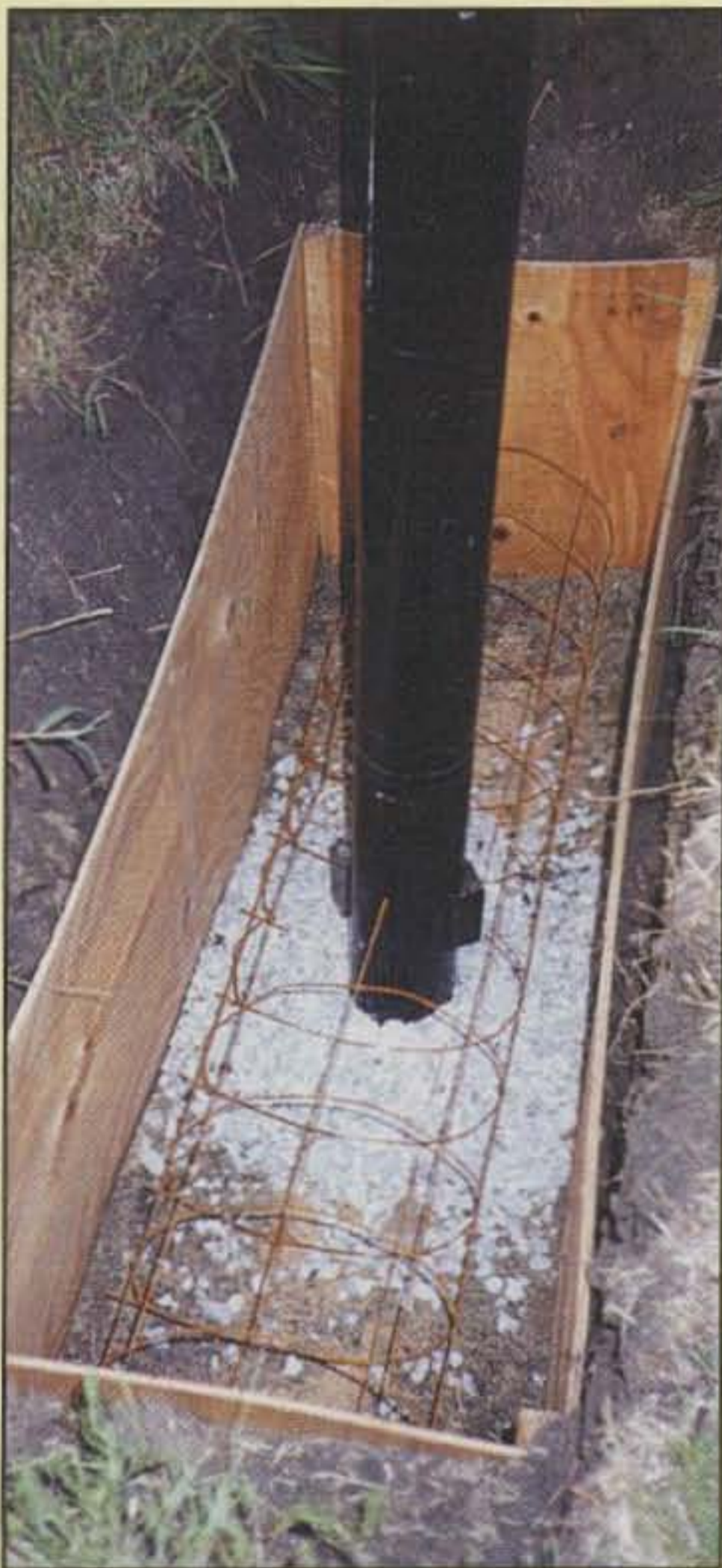
Photo C— The formed base hole with the wire mesh, sand, pea gravel, and the pole.
