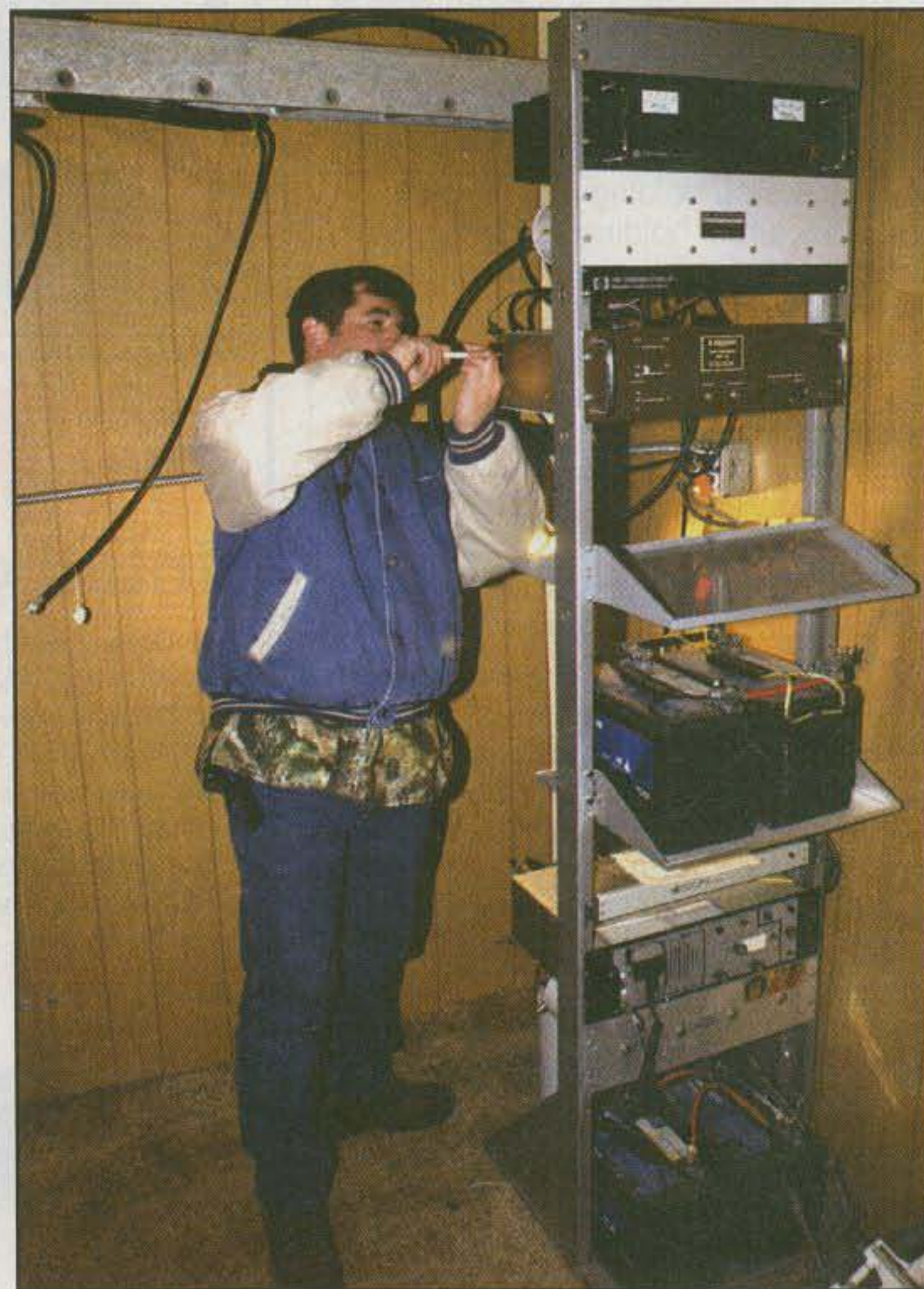
Somebody owns, and maintains, every amateur radio repeater, so when you use a repeater, act like an invited guest at someone else's station. You are! Here Andy Gagliardo, N7SGV, works on the K17D repeater overlooking Las Vegas, Nevada. (Photo by Larry Mulvehill, WB2ZPI)
