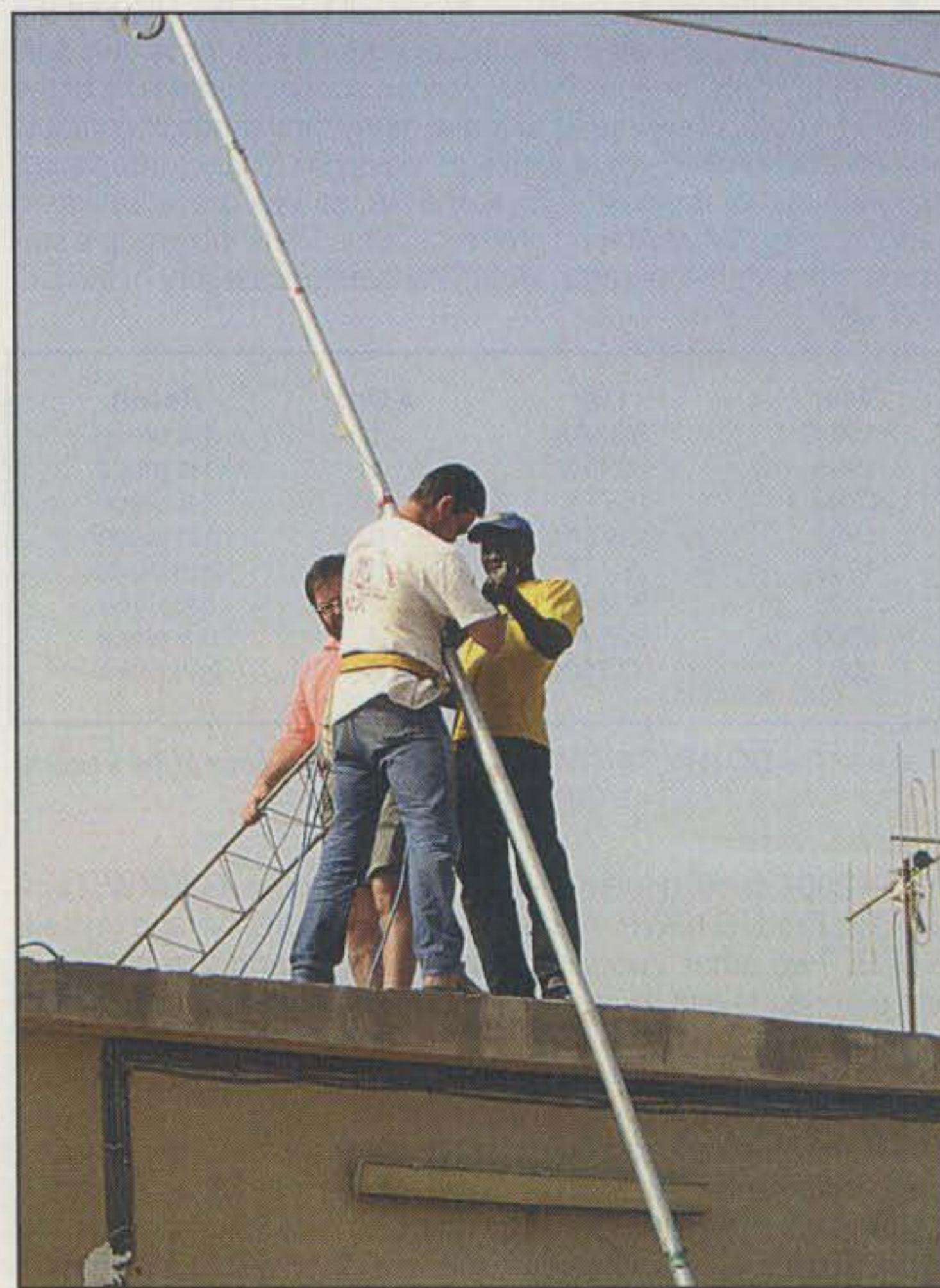
Final assembly of the 40 meter beam by Fred, G4BWP, Mike, KC7V, and Mahmud #1.
