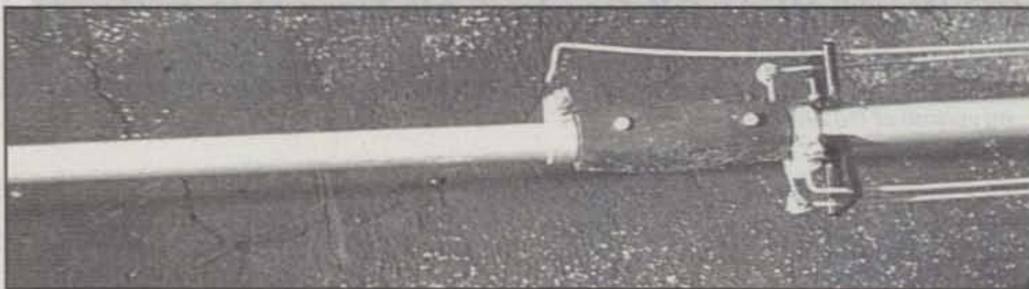
Photo A— Broken aluminum loading segment spanning the center insulator.
